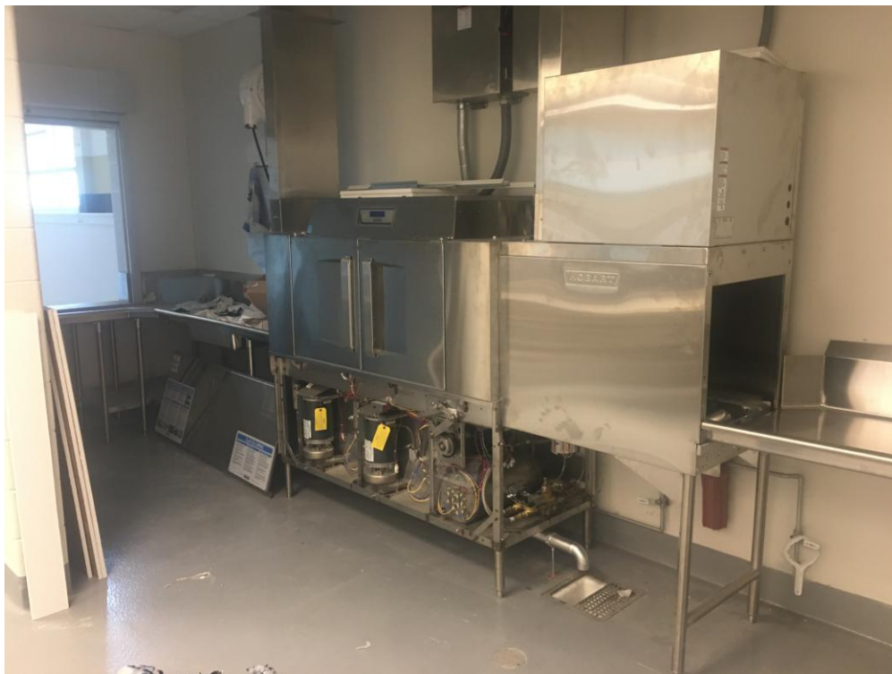
View of new Dish Machine..
