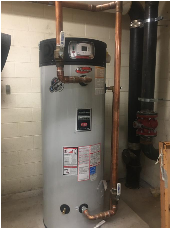
View of one of the new hot water heaters.
