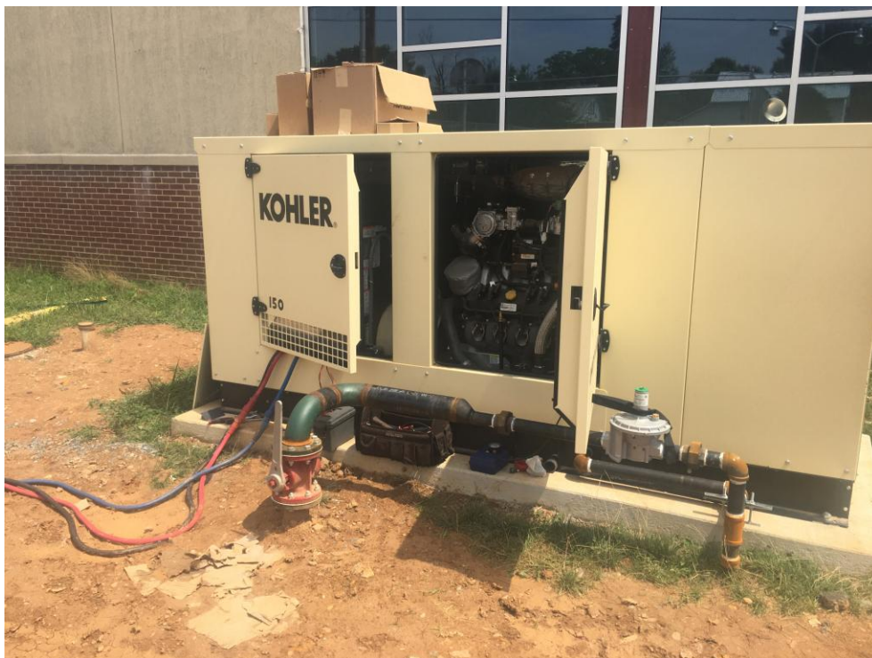
View of new Generator being load tested.
