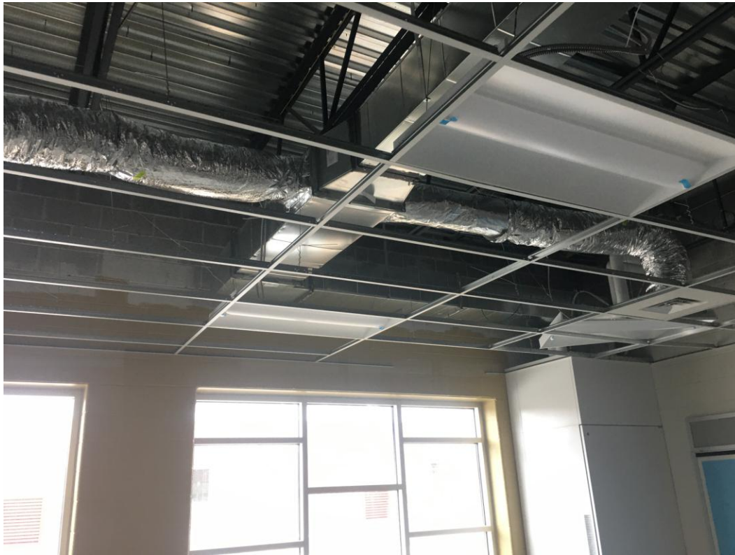
View of new light s and ceiling grid in Classroom Addition.
