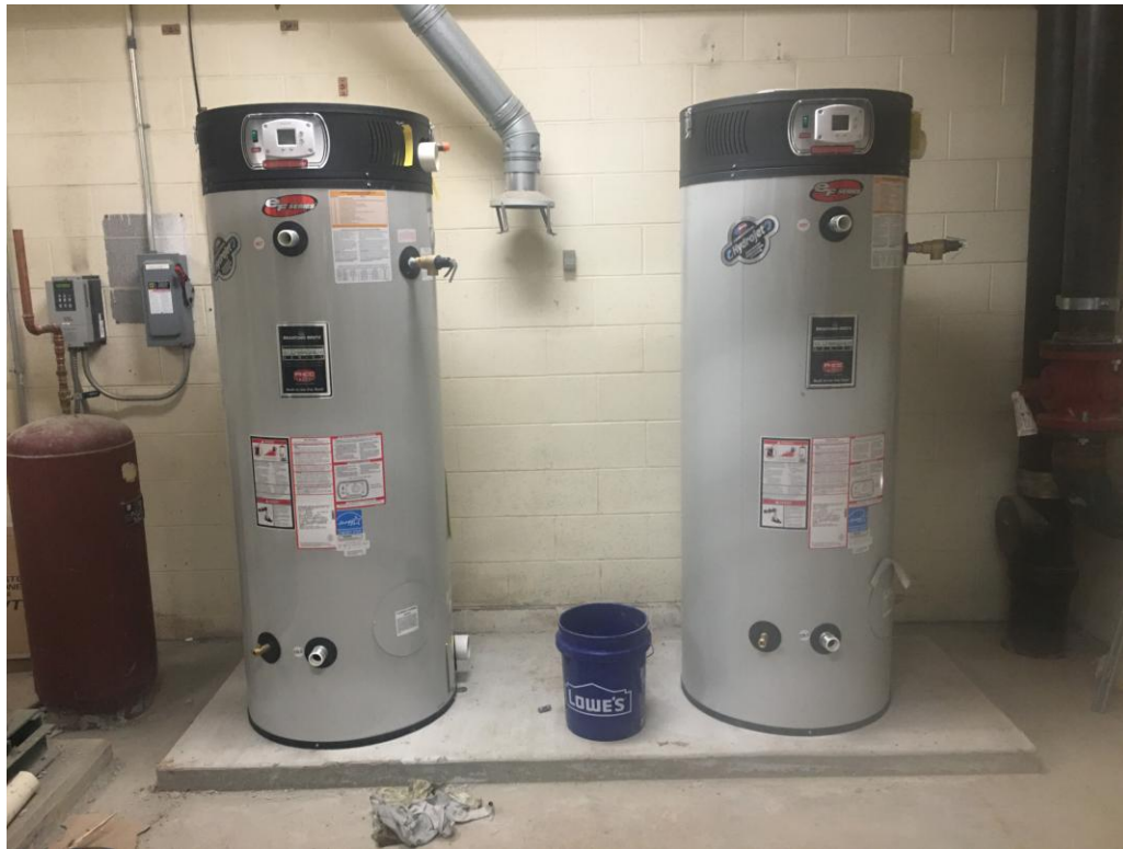
View of new Hot Water Heaters.
