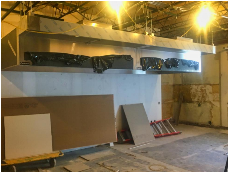
View of new Kitchen exhaust hood.
