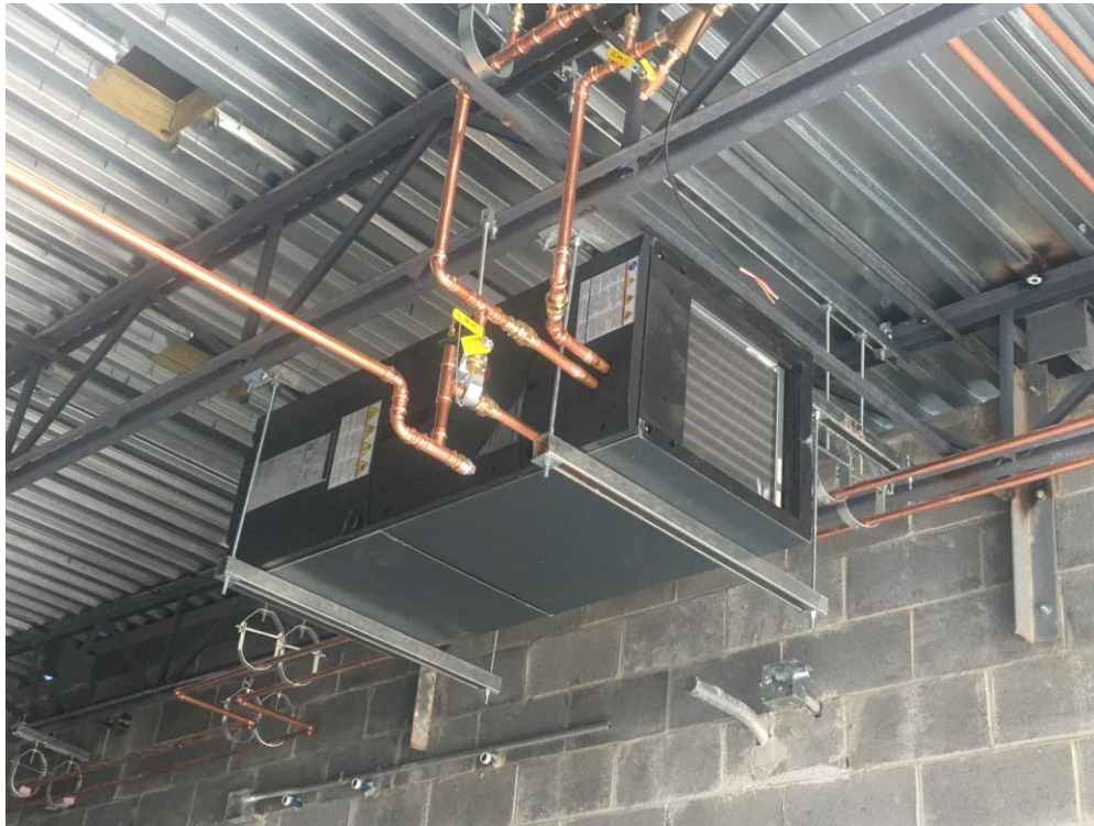
View of new air handling unit in Gifted Room in the Classroom Addition.
