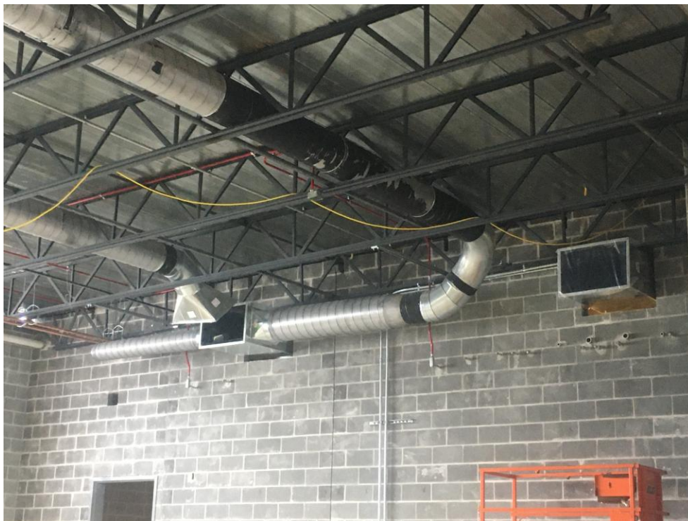
View of new ductwork in Band Room/Platform.
