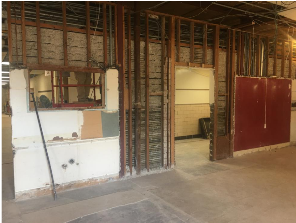
View of walls in Administration area that will need to be recovered.
