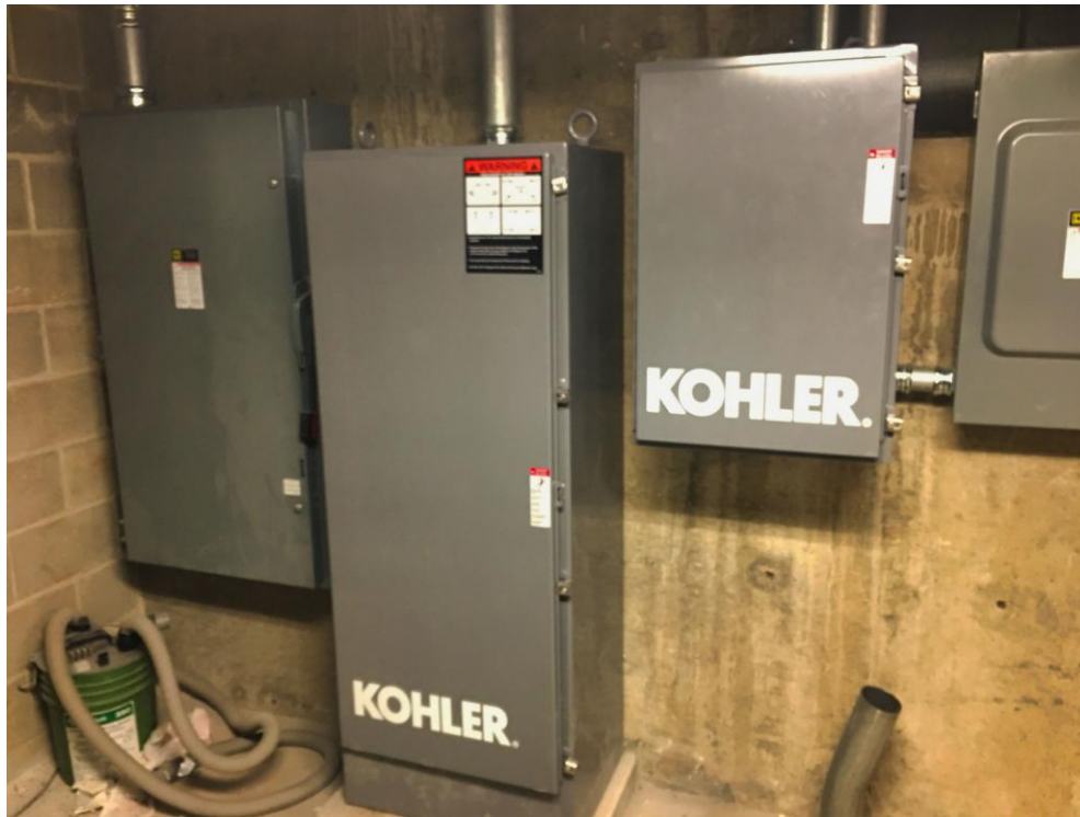
View of new Emergency Transfer Switch in existing basement.
