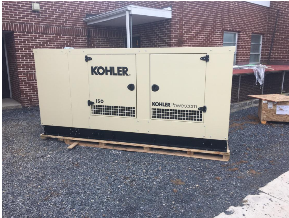
New Emergency Generator.
