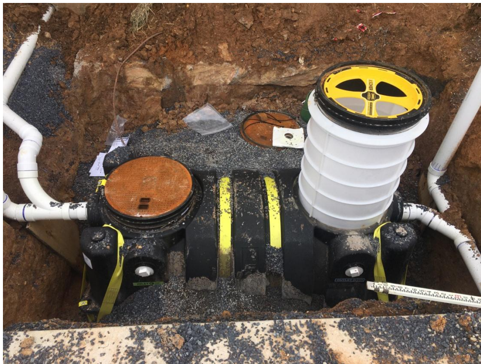
View of new Kitchen Grease Trap.
