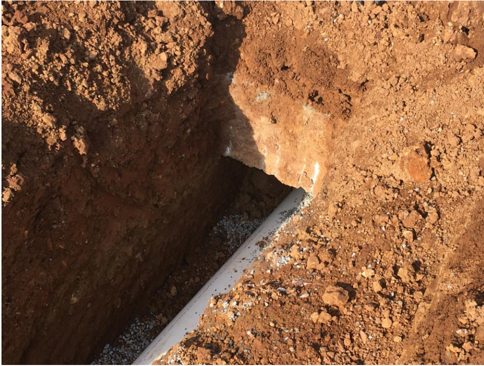
Main sewer line going under electrical duct bank, prior to exiting the building.
