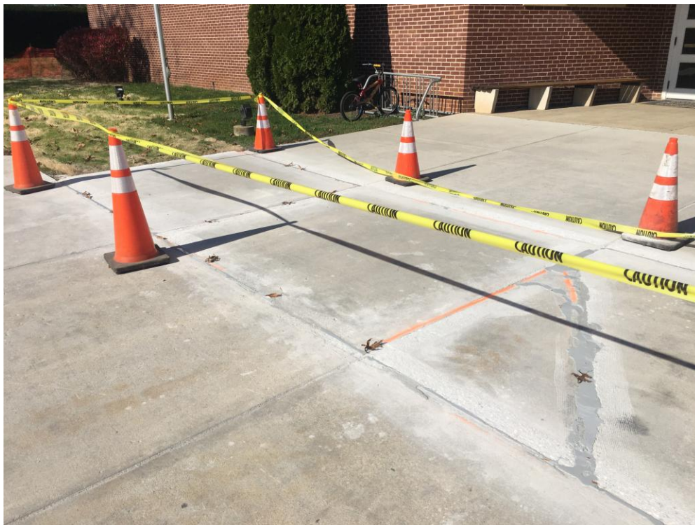
Area of sidewalk that heaved after grinding.
