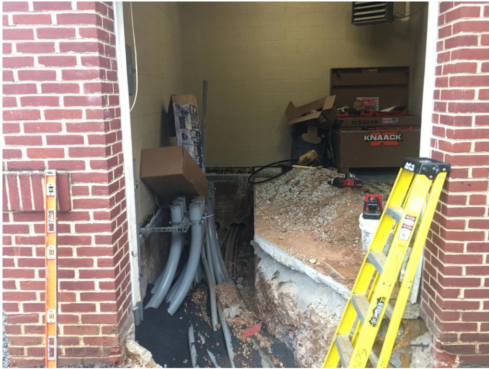
Conduits in new Switchgear Area.
