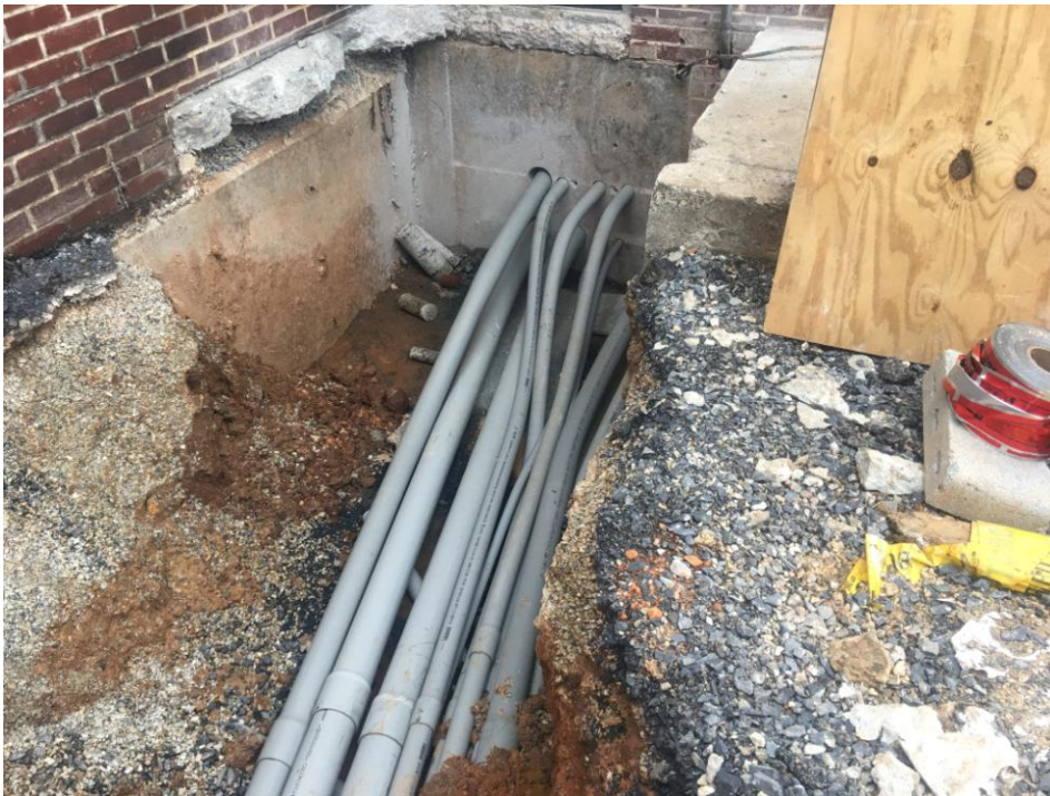
Duct Bank into basement Mechanical Room.
