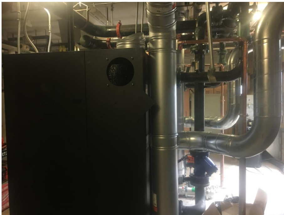
View of new breeching on new BES boilers.
