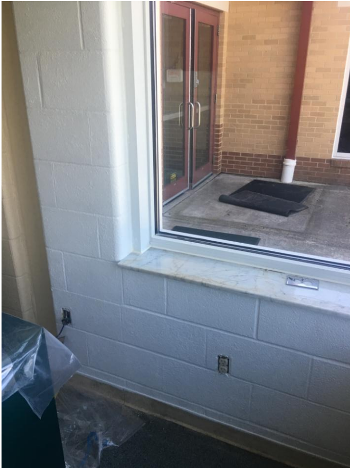
View of wall that was repainted at BES due to water infiltration around old window.
