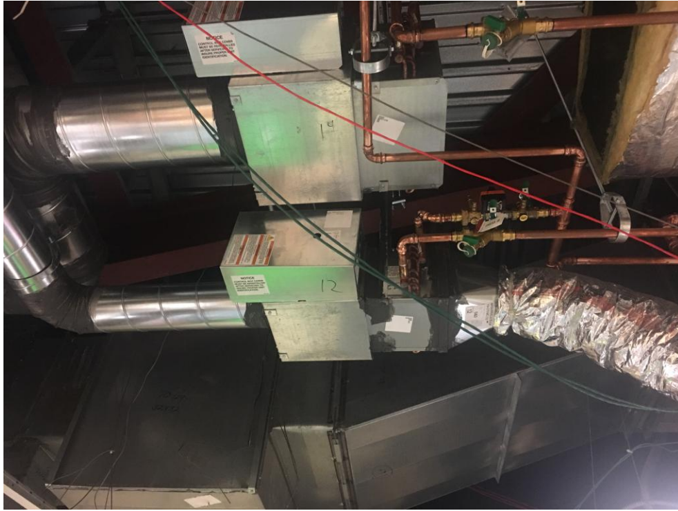
View of reheat coils in ductwork at BES.
