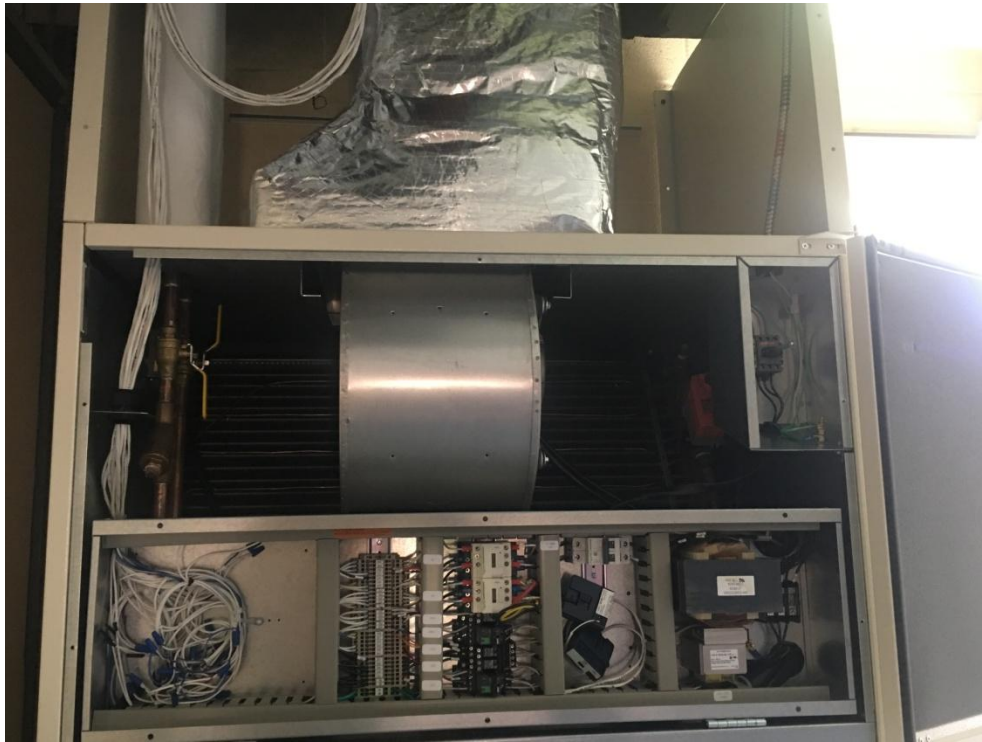
View of Top of classroom VUV showing control wiring and supply fan.
