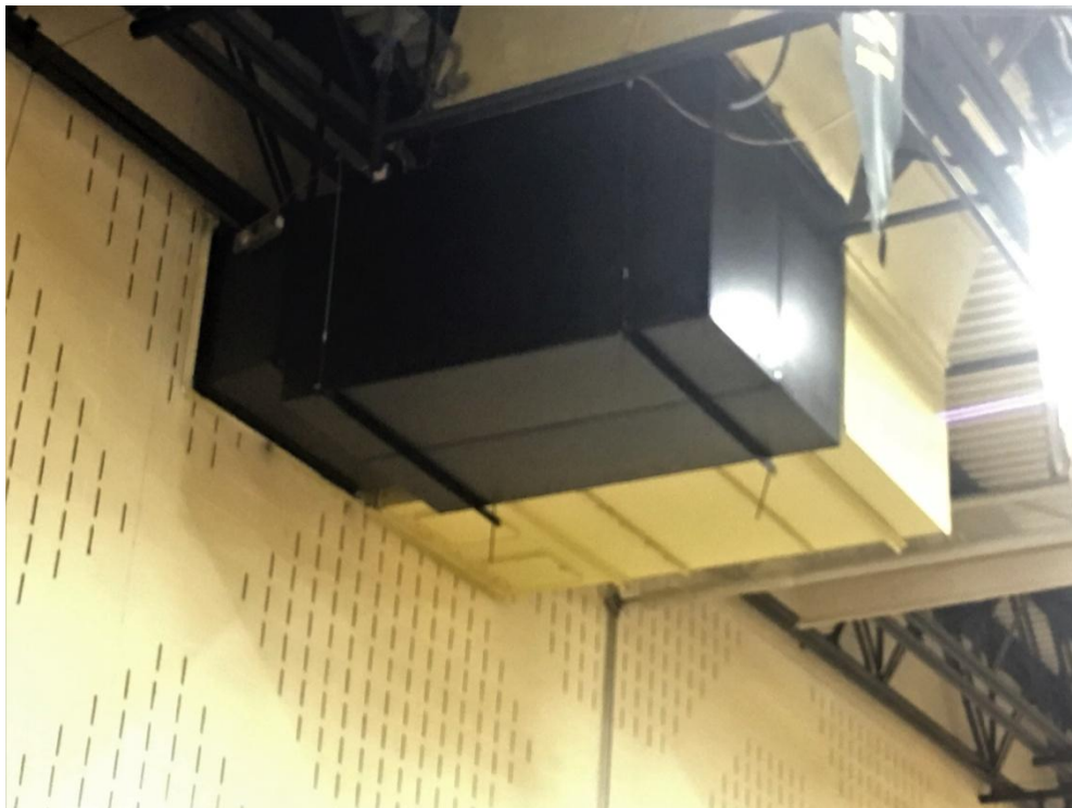
View of new return ductwork in BHS gym.
