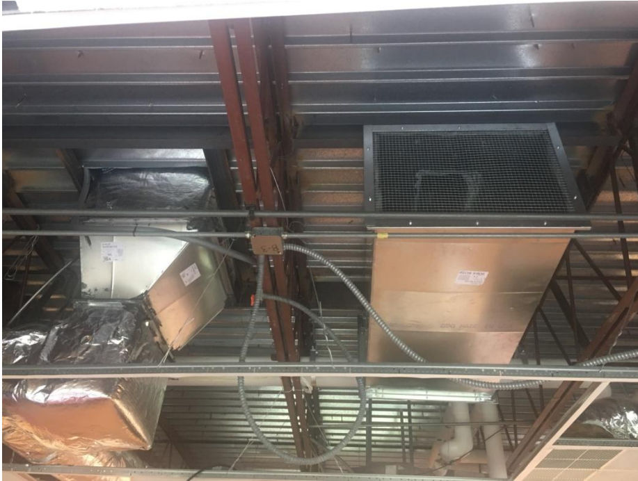
View of rooftop unit duct connections at AES Library.
