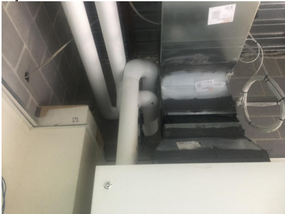
View of piping into VUV after insulation.
