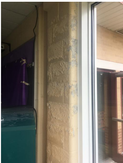
View of wall efflorescence at BES from old window leak.
