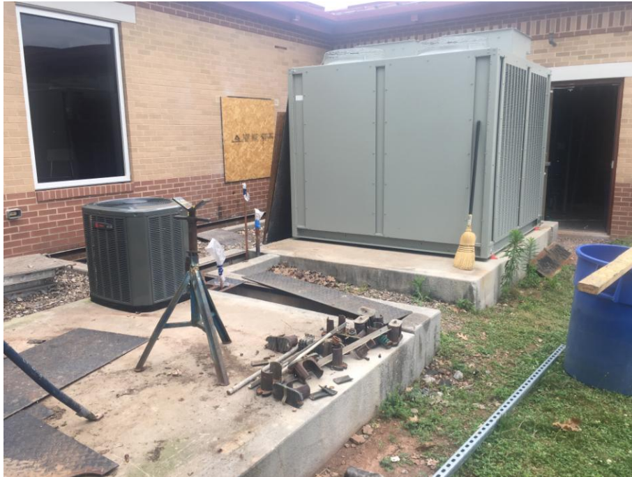
View of new condensing units at BES.
