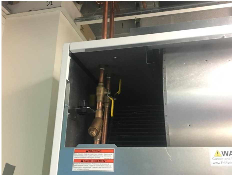
View of plumbing connections to VUV unit at AES.
