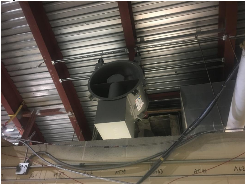
View of new Axial Return Fan RF-1 at BES.
