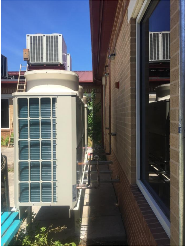
View of new condensing units at BES.
