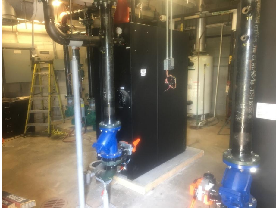
View of one of the new boilers at BES after piping installed.
