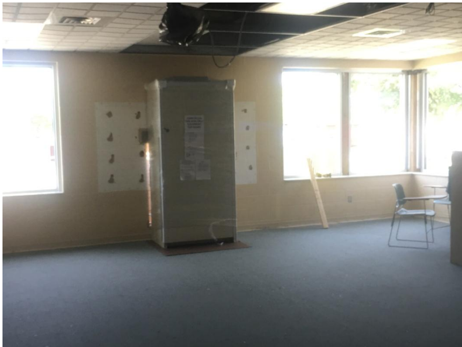
View of VUV unit in place at BES.
