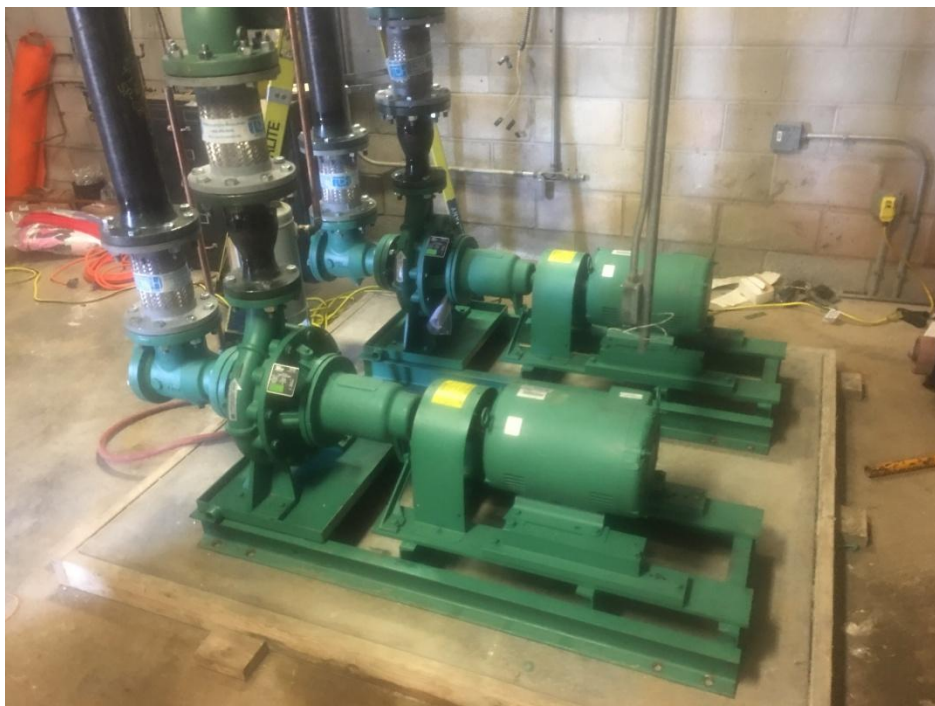
View of new HVAC pumps at BES.
