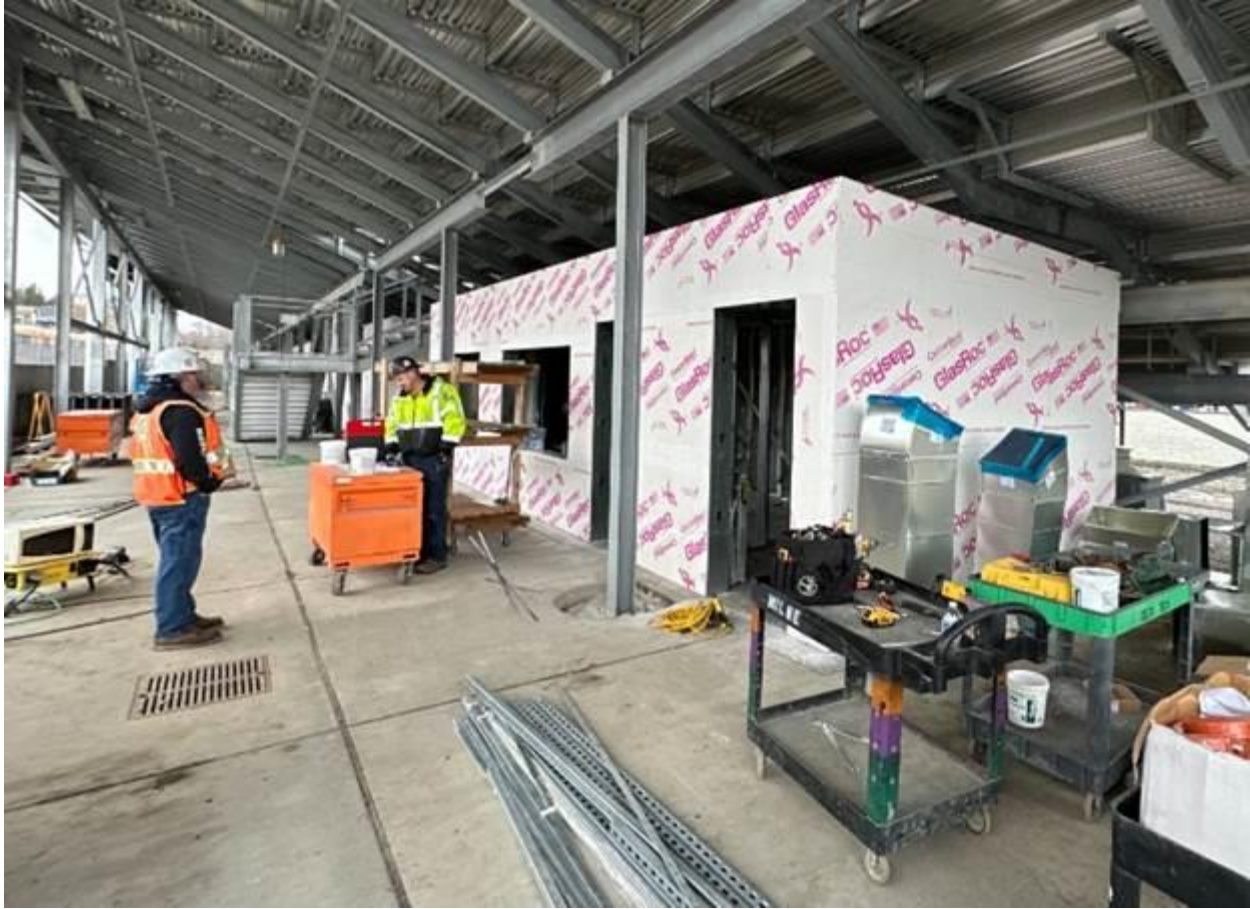
The concession area under the football field grandstands has now had framing and exterior sheetrock completed
