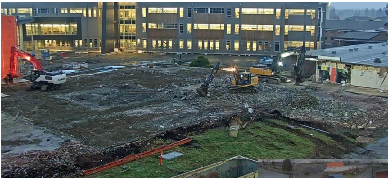
The north end of the old FHS is gone – this will allow construction of the CTE Wing to begin
