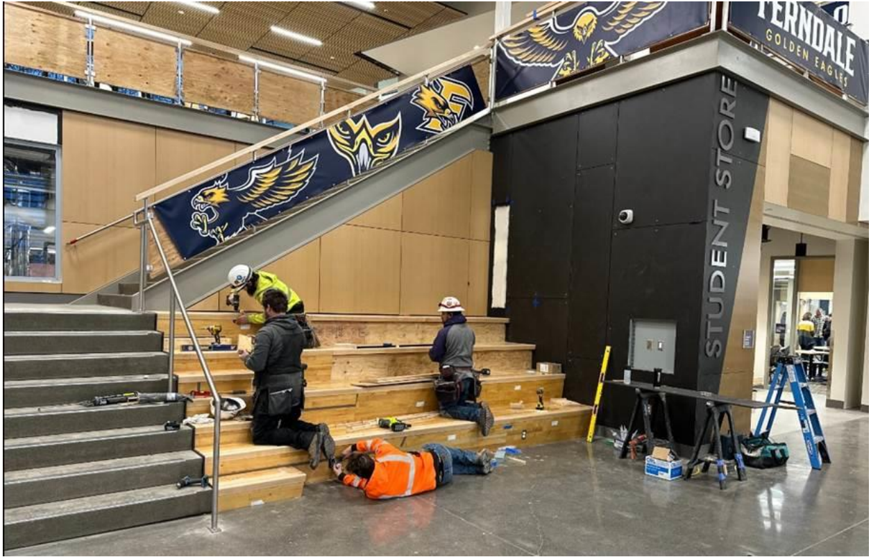
Finishing touches that were made in the Commons Area before students arrived
