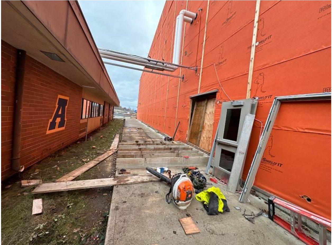
The temporary entrance to the Athletic Wing was sealed up in preparation for the demolition of the old building
