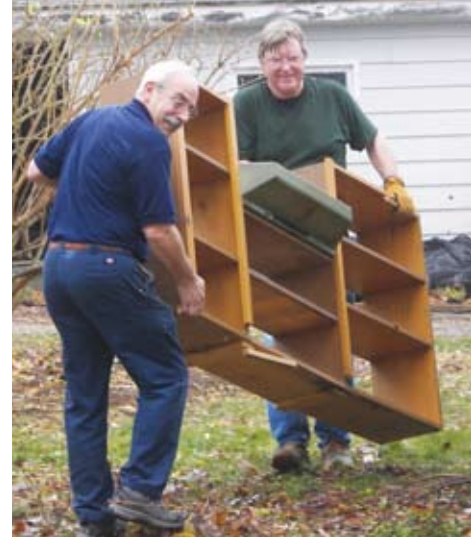
George Comeau and Gregg Hannah remove kitchen cabinets from the Beach property
