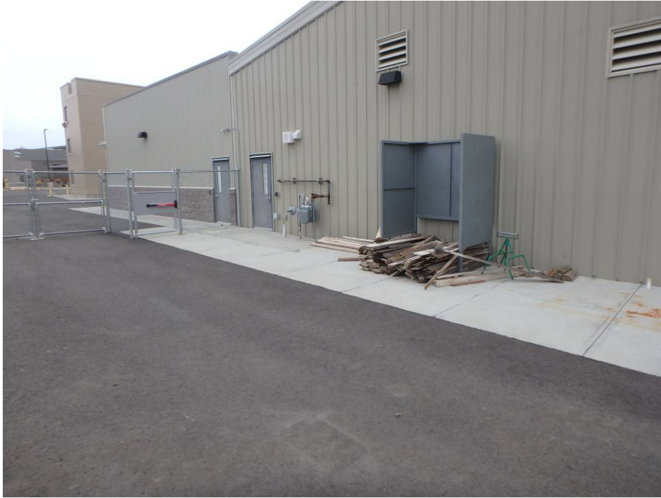
Area in front of the south elevation of Tri Tech East that will have the new gas line
