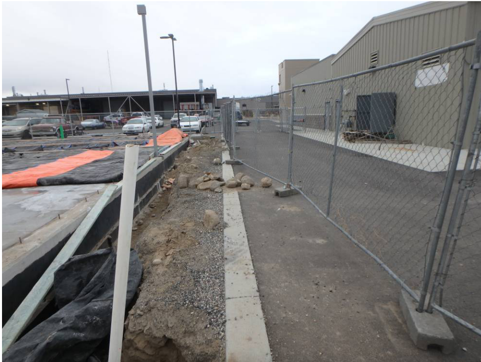
Looking west at the north end of the slab, foundation wall and column
