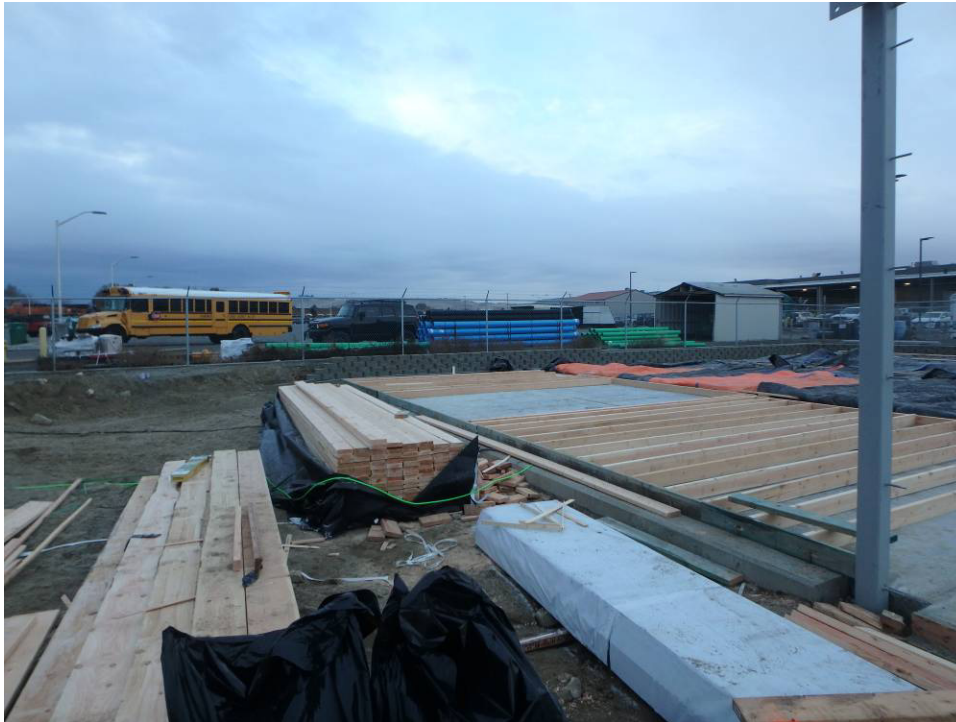
Looking south at the Southeast corner of the slab with the east wall framing
