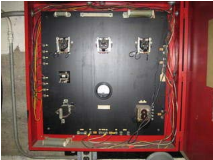
Fire Alarm System Control Panel
