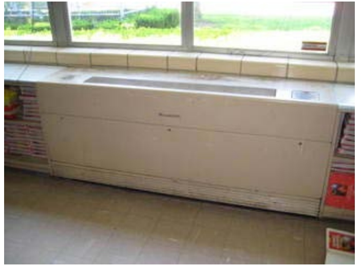
1962 Addition Steam Unit Ventilator
