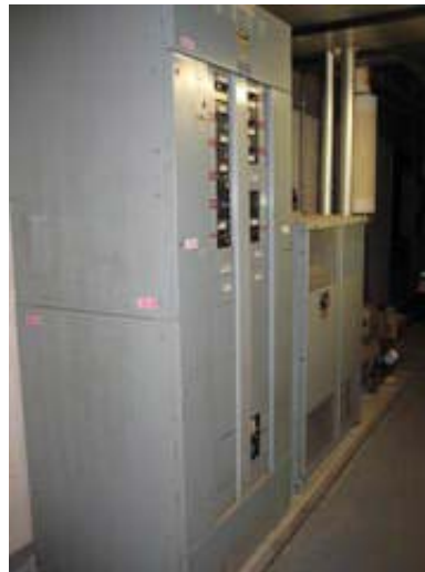
Main Electrical Distribution Panel
