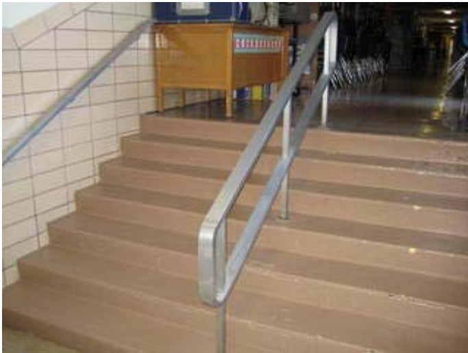
Non-Compliant Stairway and Railing
