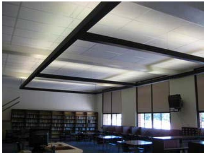
1922 Original Construction Media Center Indirect Fluorescent Light Fixtures
