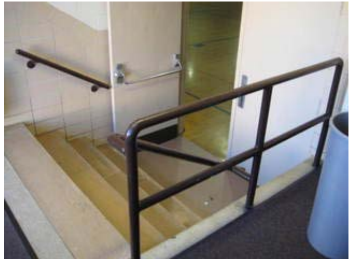
Non-Compliant Stairway and Railing
