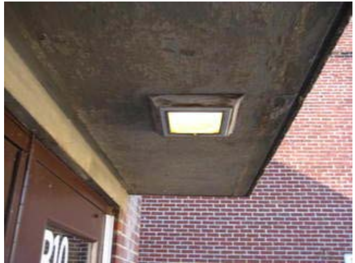
Recessed Entry Light Fixture
