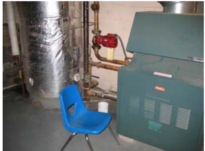
Domestic Hot Water Heater and Storage Tank
