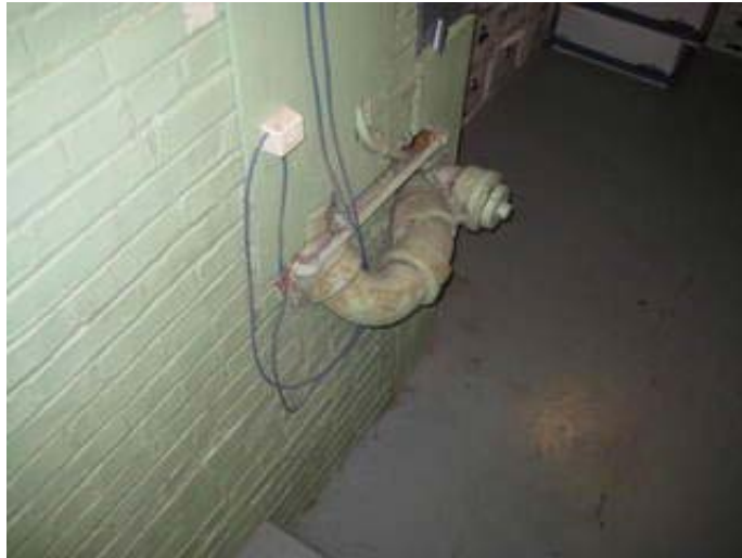
Sanitary Waste Piping
