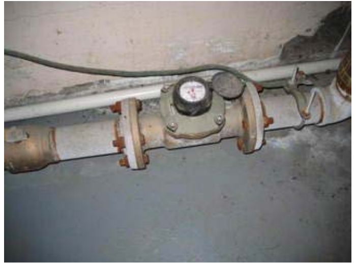
Incoming Domestic Water Meter
