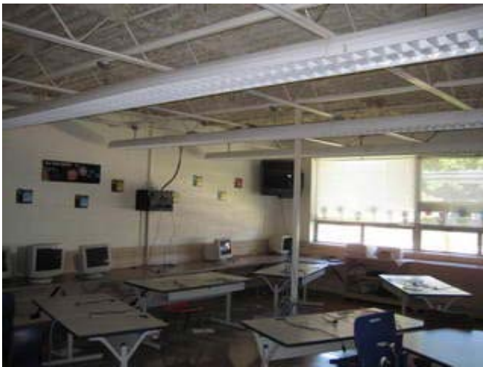
1962 Addition Classroom Fluorescent Light Fixtures
