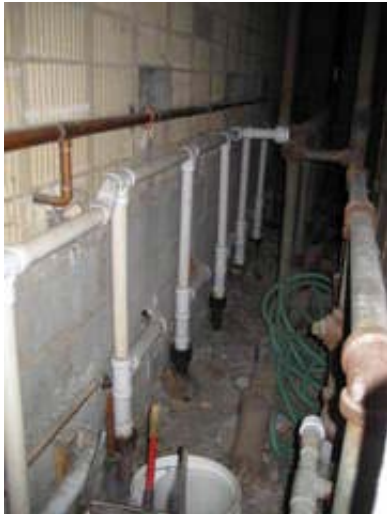
Sanitary Waste Piping
