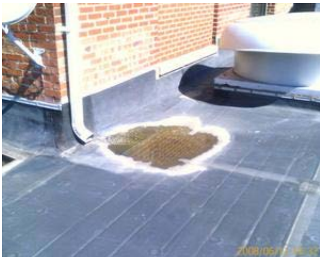
Typical Standing Water Condition
