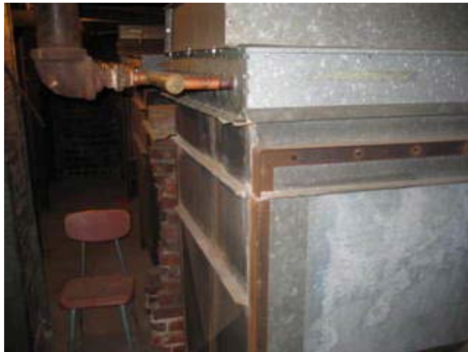
1922 Original Construction Air Handler
