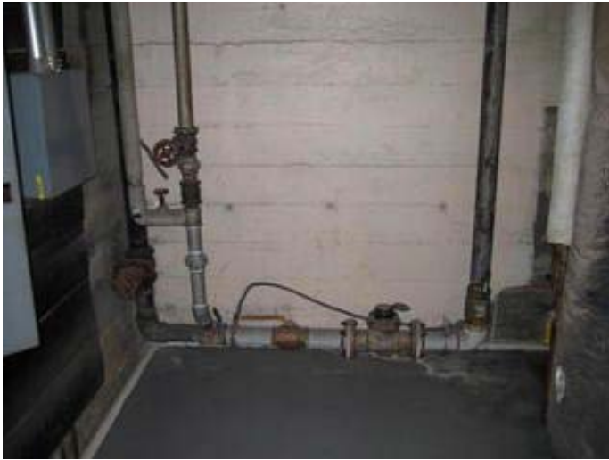
Incoming Domestic Water Service
