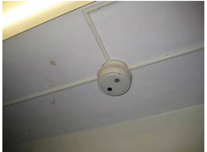
Fire Alarm System Smoke Detection Device
