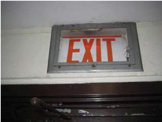
Non-Compliant Non-Illuminated Exit Sign
