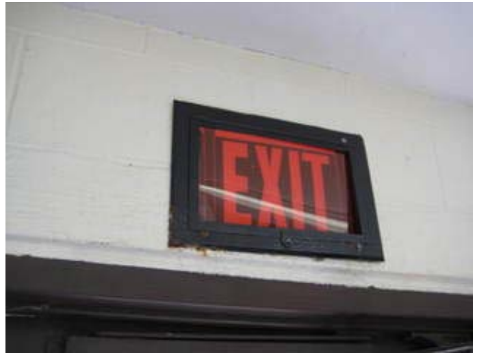
Non-Compliant Exit Sign
