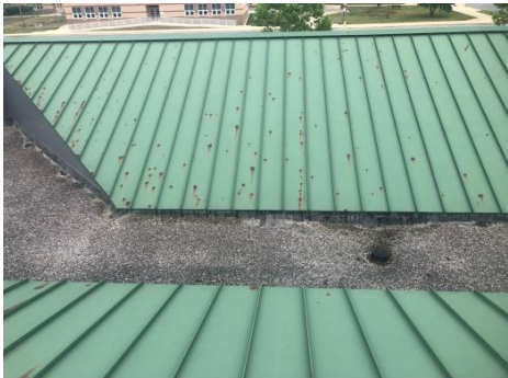
Roof is in fair condition. The metal roofing needs painting or pm
