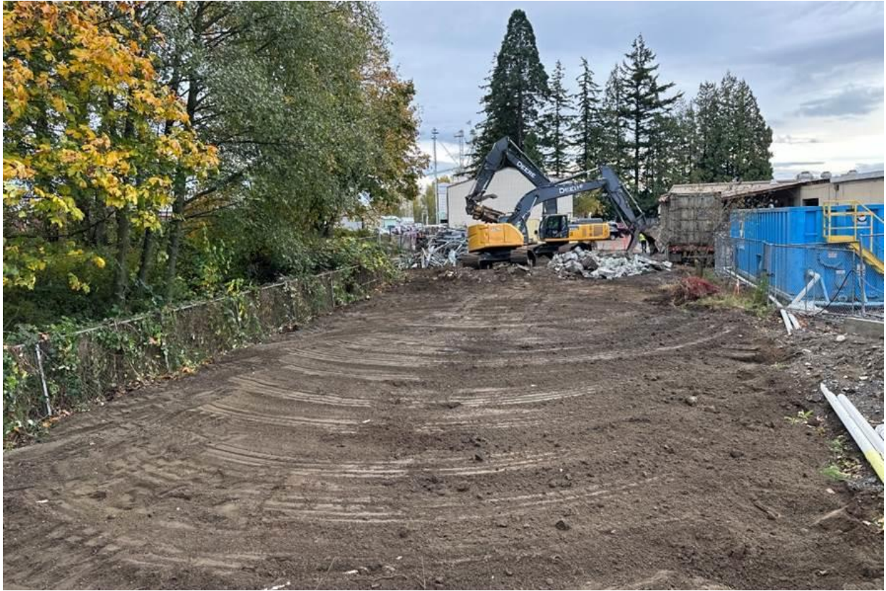
The old Aquaculture Building is gone! Crews will now start prepping this area for the Emergency Generator.
