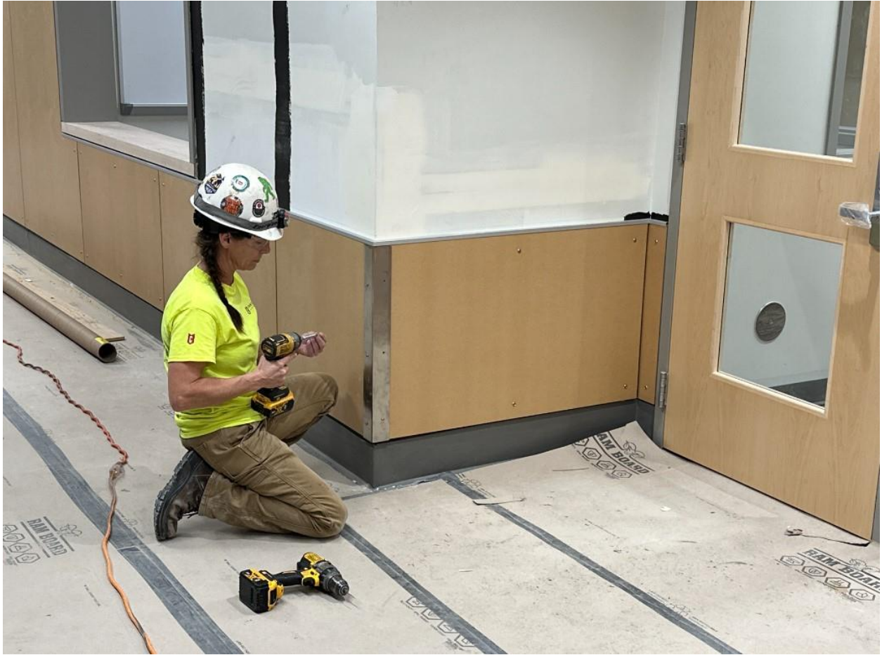
Finishing touches like corner guard installations are happening in the Academic Wing
