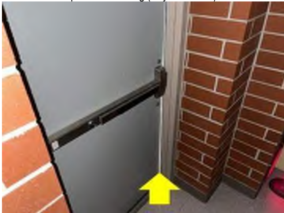
Door Weather-Stripping – weather-stripping was improperly installed at the sides of the door as seen by clear daylight at the perimeter of the door (Spring-Ford Area HS).
