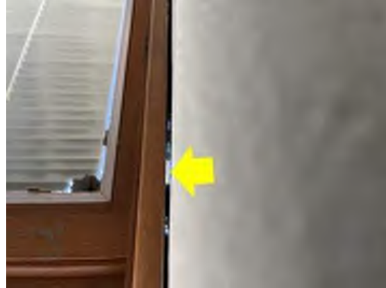
Caulking – missing sealants at the window casing are leading to a clear air leakage pathway as seen by daylight (Limerick ES).
