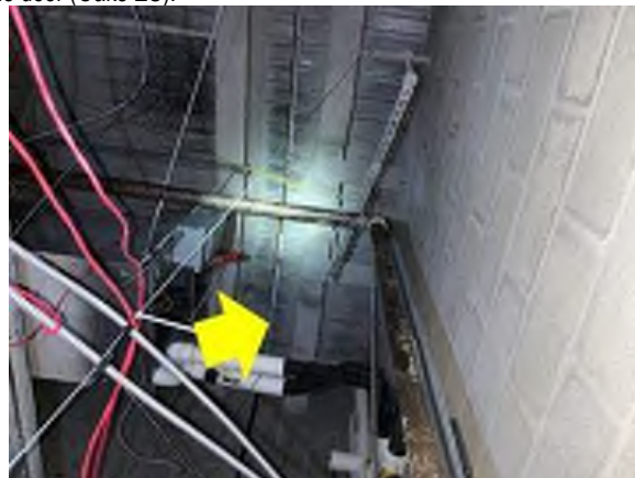
Roof Insulation – roof assemblies were connected but insulation is not continuous. It is believed that condensation forms at these intersections and drips onto drop ceiling below; enhancing the thermal barrier (5th-7th Grade Center).
