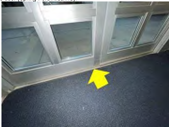
Door Weather-Stripping – a missing door sweep next to an existing door sweep needs to be installed to prevent drafts at the bottom of the door assembly (Royersford ES).
