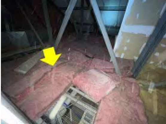
Attic Air Barrier Retrofit – chicken wire supporting unfaced fiberglass is a building envelope flaw. Dirt build-up at fiberglass intersections is a clear sign of air permeable fiberglass “filtering” air leaking through the thermal envelope of the building (Royersford ES).
