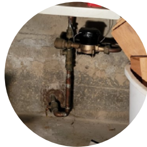
This is an example of a water meter.
