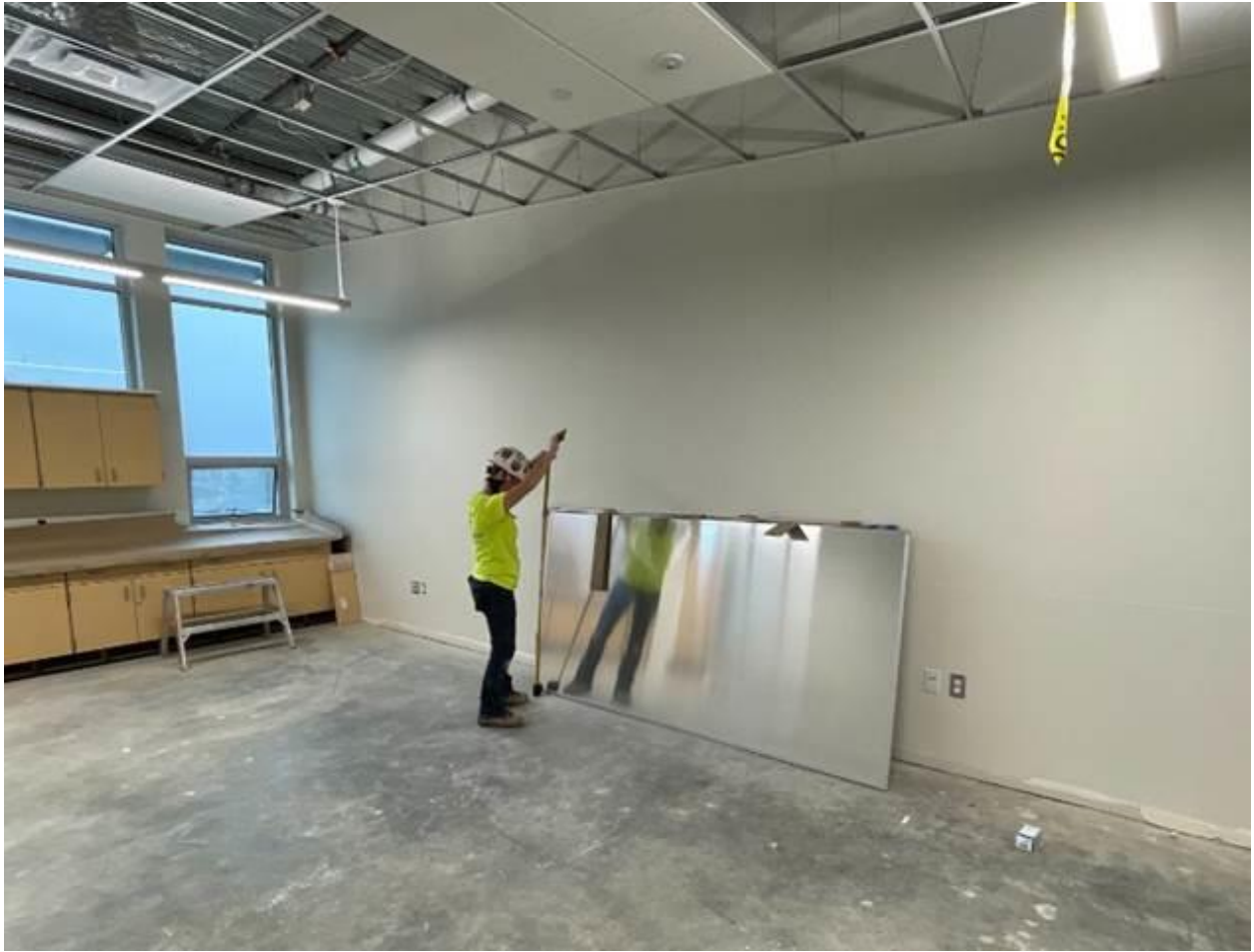
Whiteboard installation in the Academic Wing
