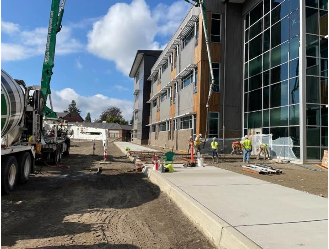
Final sidewalks being poured in the staff parking area south of the Academic Wing
