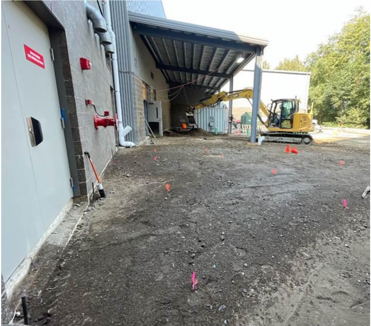
Final prep work in the service yard east of the kitchen area
