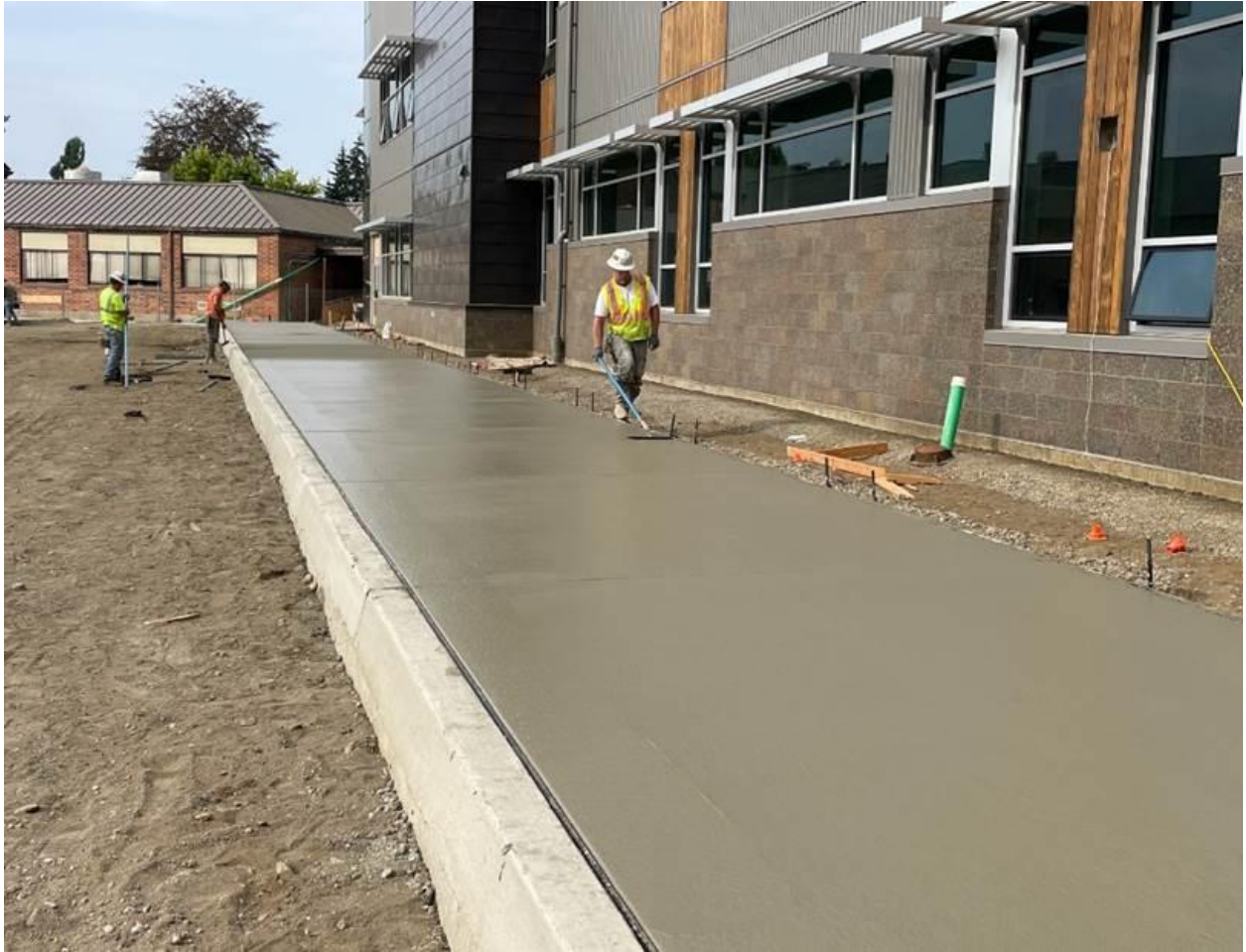
Pouring of sidewalks around the staff parking area south of the Academic Wing
