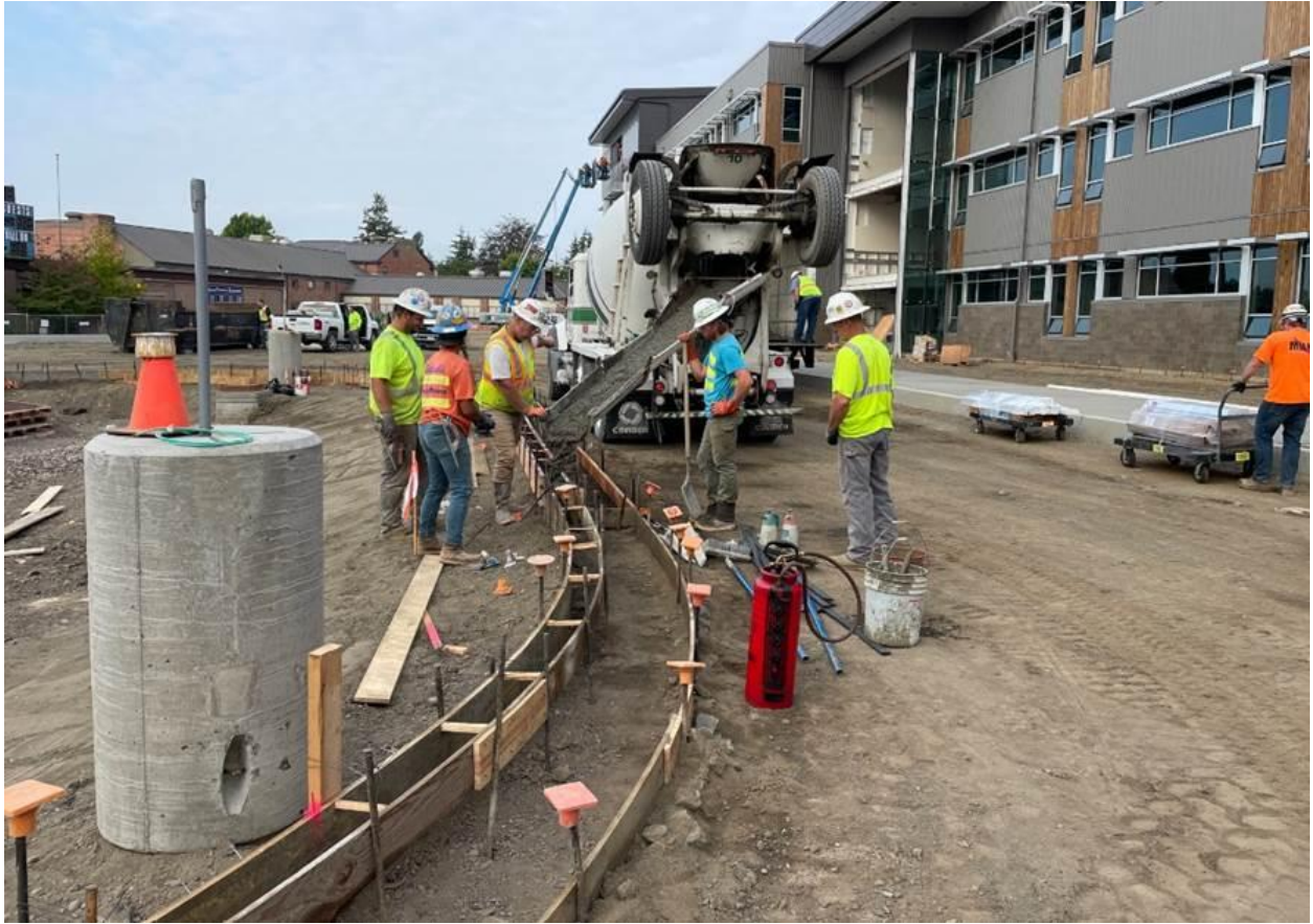
Pouring of curb and gutters around the staff parking area south of the Academic Wing
