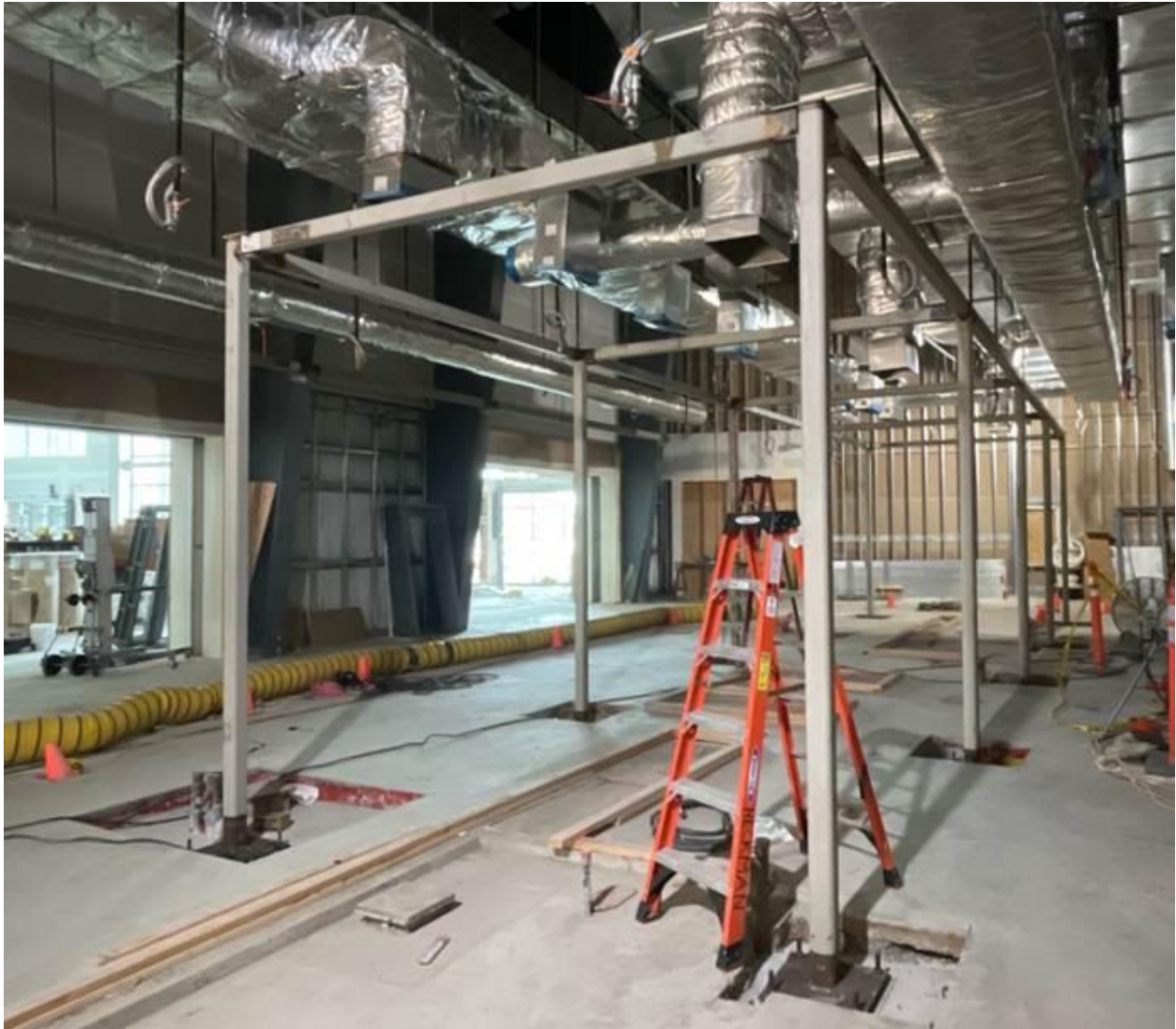
Substructure installation in the kitchen area. This structure will support the kitchen hoods, ceilings, lights and fire sprinkler system.
