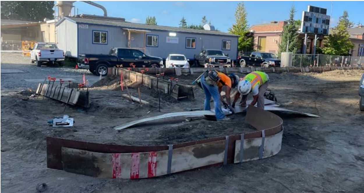
Curbs and gutters being formed at the staff parking area south of the Academic Wing
