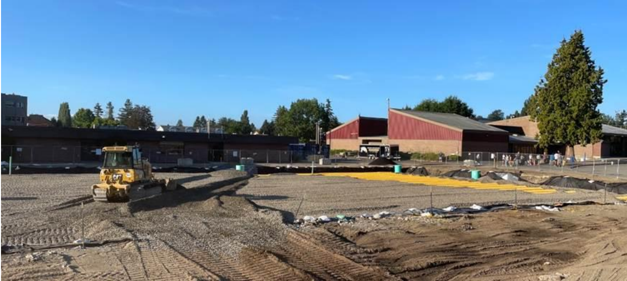
Underwater stormwater storage system on the north side of the new gym receiving its final topping of gravel
