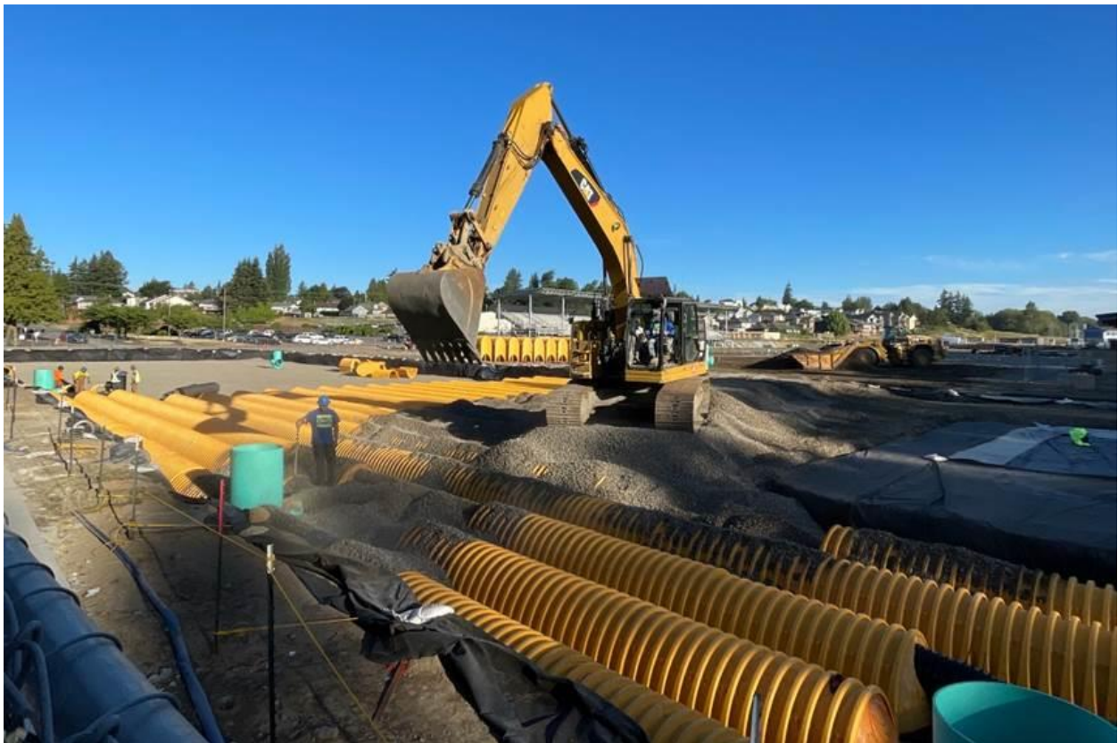
Final installation of the underground stormwater storage system on the north side of the new gym
