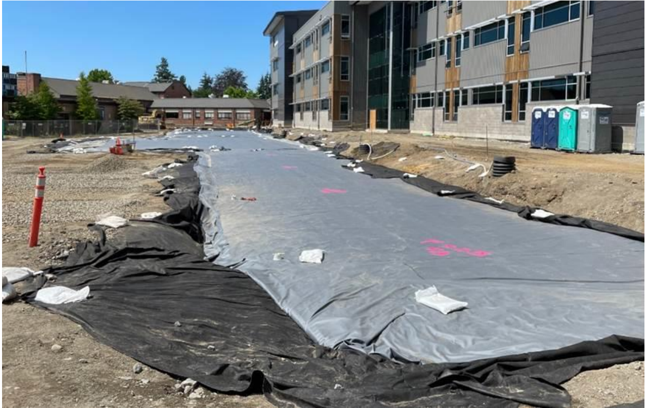
Underground stormwater detention system on the south side of the Academic Wing is complete
