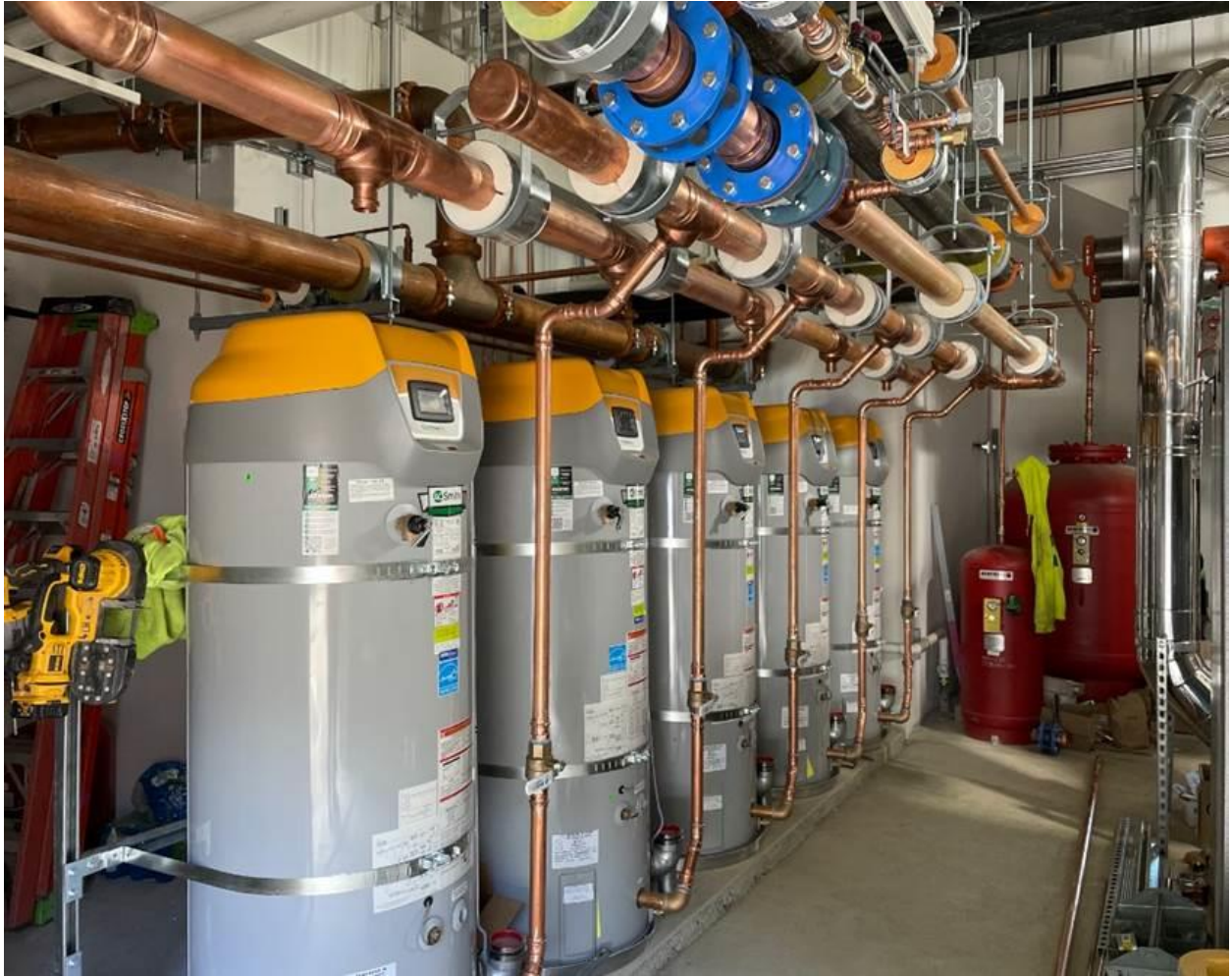
Commercial hot water heaters in the boiler room
