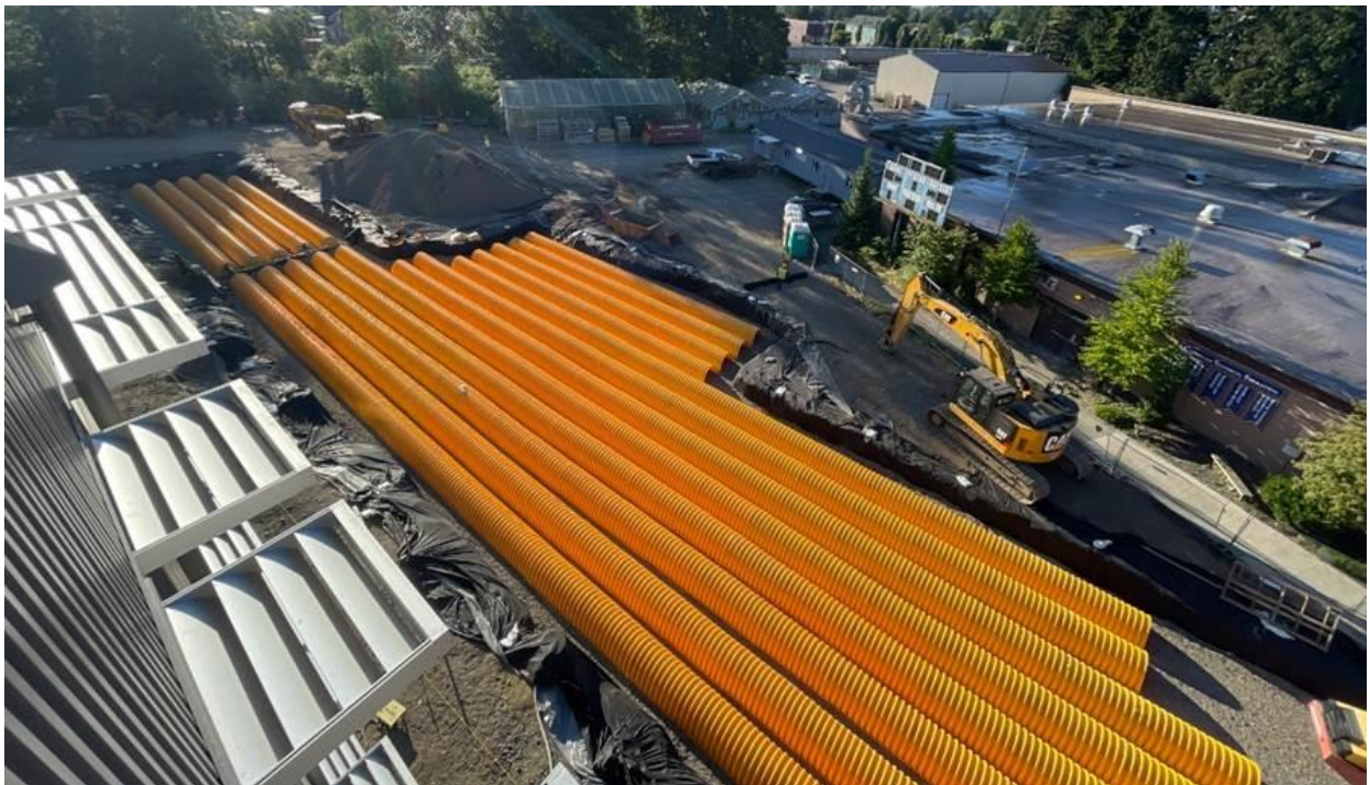
Underground stormwater detention system at the south end of the Academic Wing
