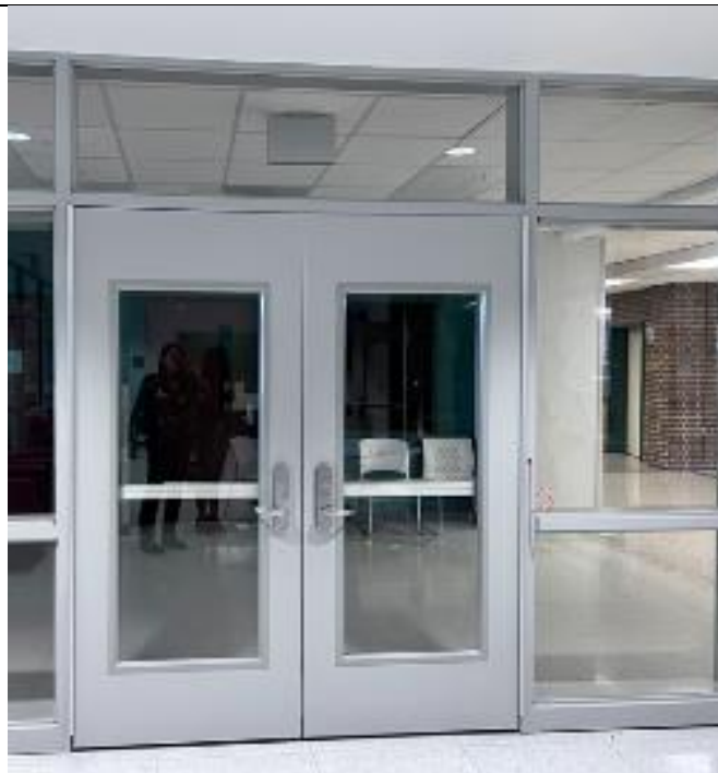
Existing lobby doors are painted and ready to have card reader installed.
