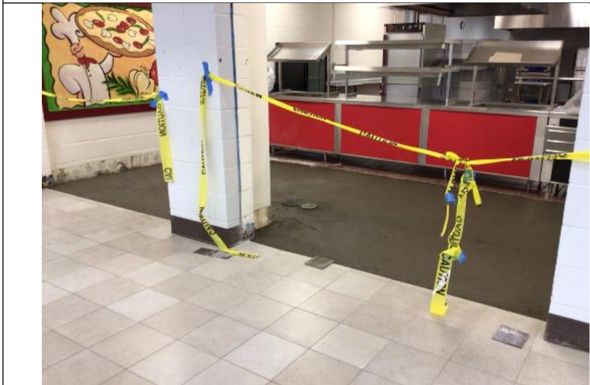
Quarry tile is being installed at the Pizza Scullery room. Doors to be installed soon.
