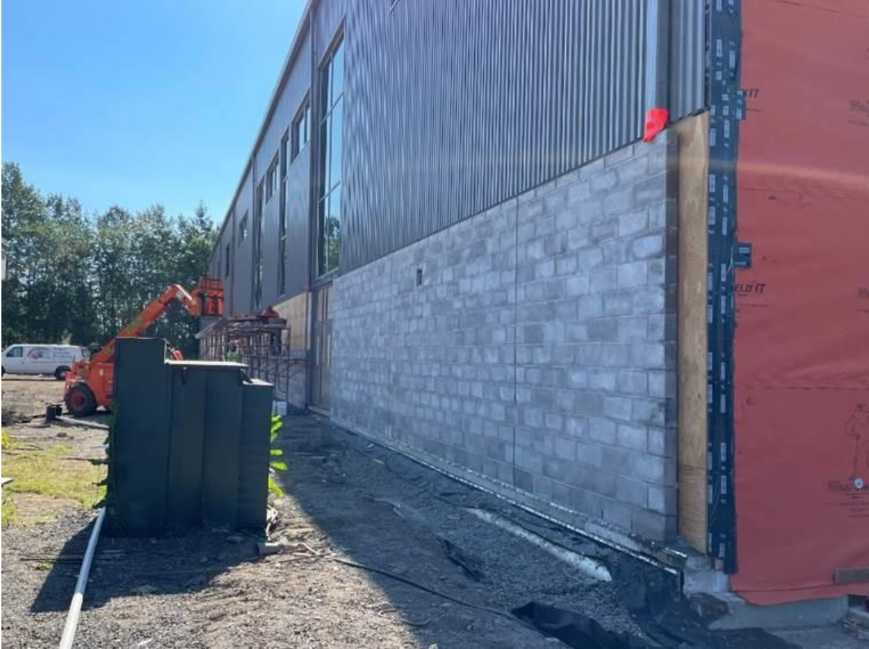
Masonry Block making good progress on the north side of the gym
