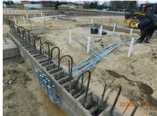
Underground electrical piping in Unit A
