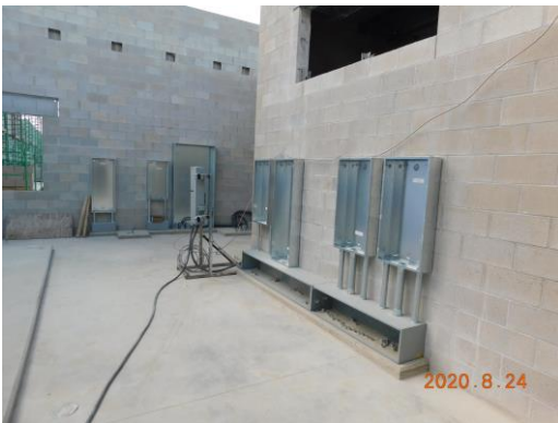
Electrical panels in Unit C
