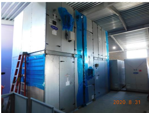
Air handling equipment placed in the Unit B mezzanine
