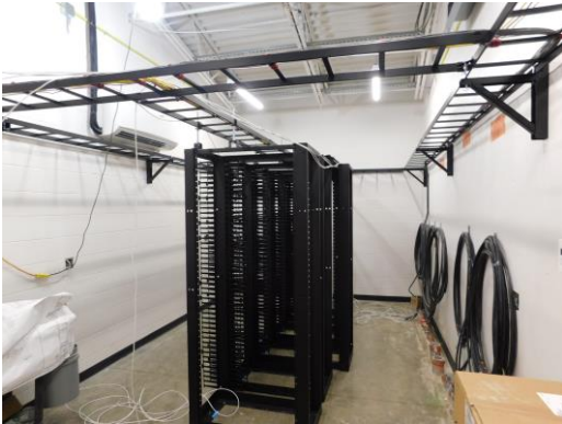
Tech room racks and ladders installed in the main tech room
