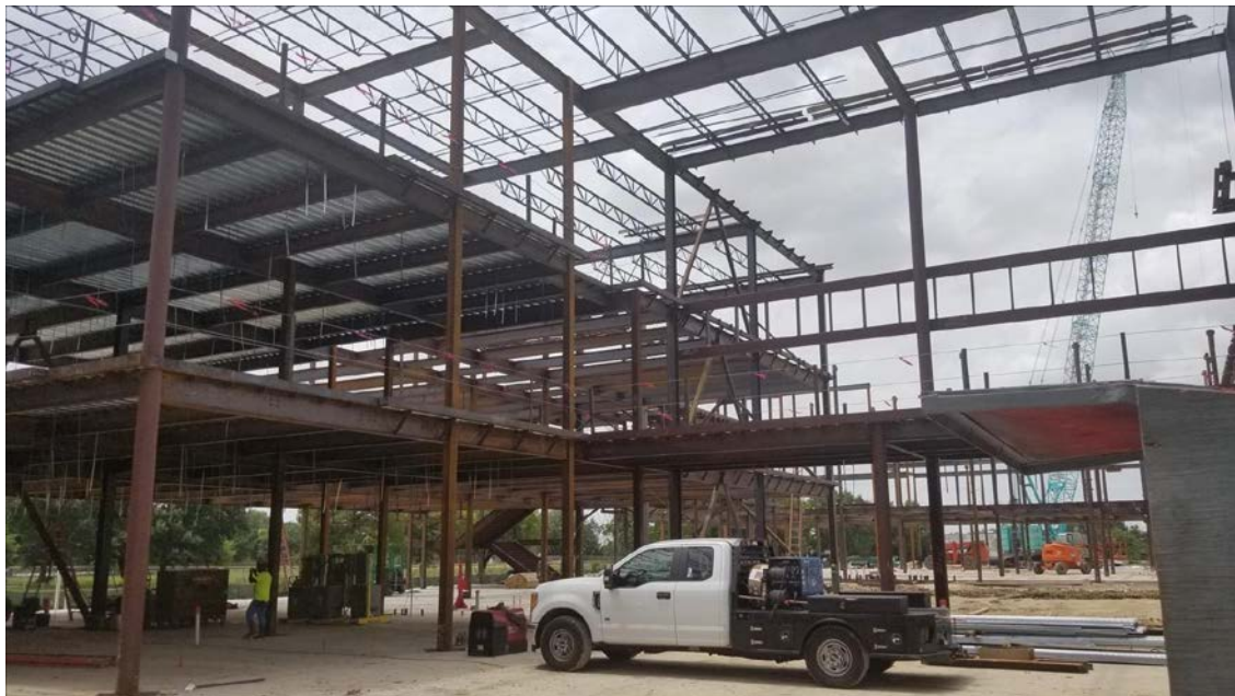
Steel Erection Area A with joists and decks, Area B and C steel beyond – June 30th
