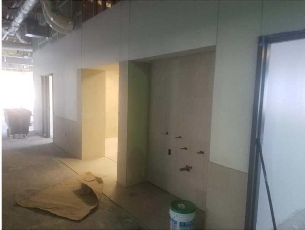
Drinking Fountain Location at Student Restroom
