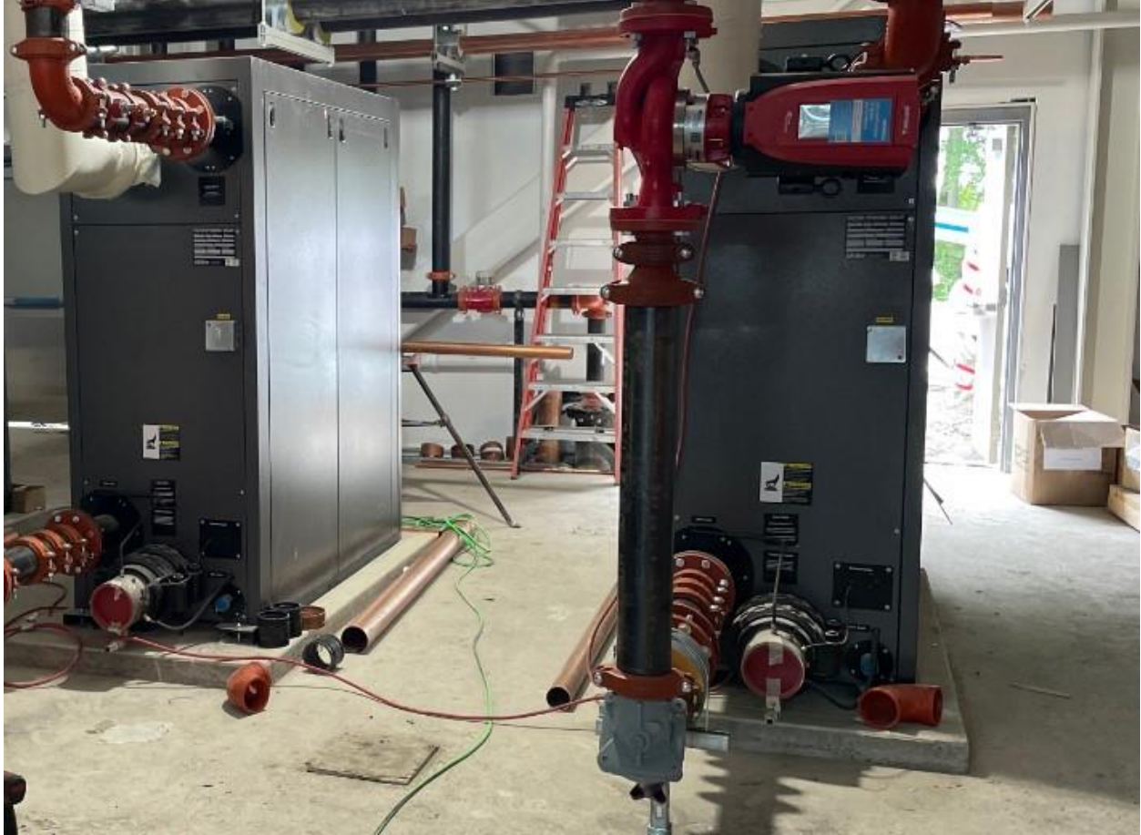
A couple of the water boilers that will provide hot water to the heating system
