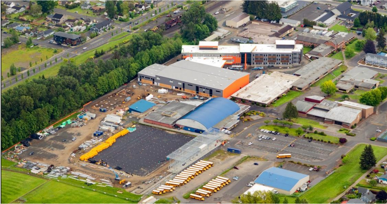
...and this is our aerial project photo from June 2022. Facing many challenges over the winter, our contractors have done a great job getting past those hurdles and making this much progress while staying on schedule. Great job to all of our crews working on the project!
