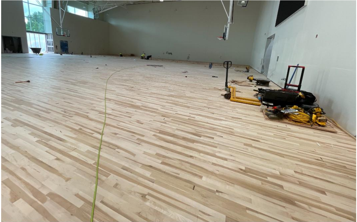
Wood flooring installation in the Main Gym is just about wrapped up
