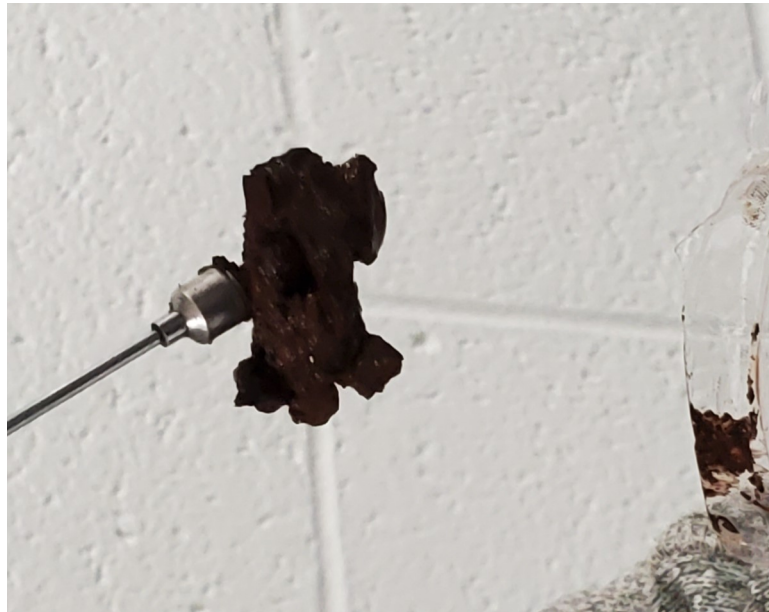
Iron deposits in glycol loop
