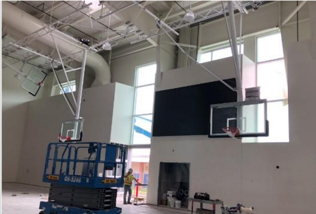
Large electronic scoreboards in the Main Gym are installed
