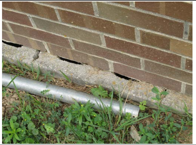
Photo 8 – Exposed cells of block foundation along South Elevation
