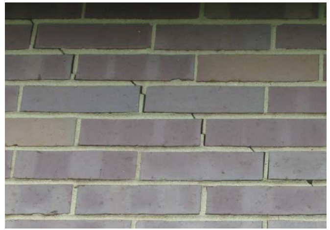
Photo 10 – General shrinkage cracks in brick veneer
