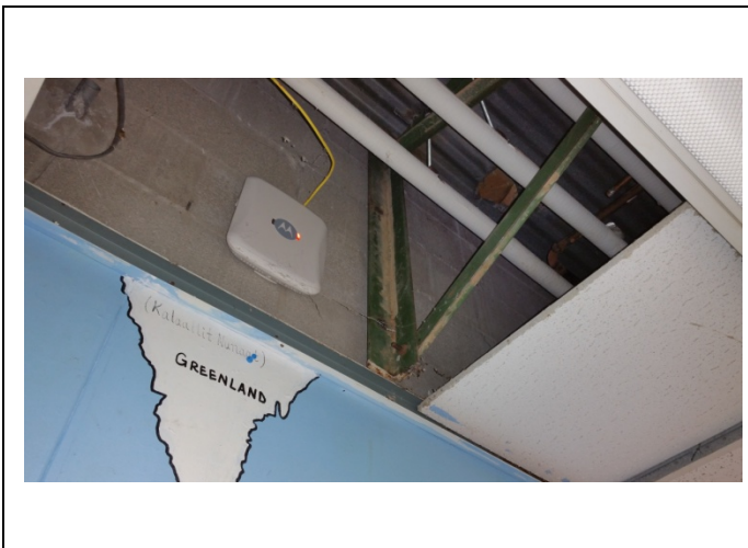
Photo 5 – Typical Bridging Angle with Missing Anchorage Bolt to Wall
