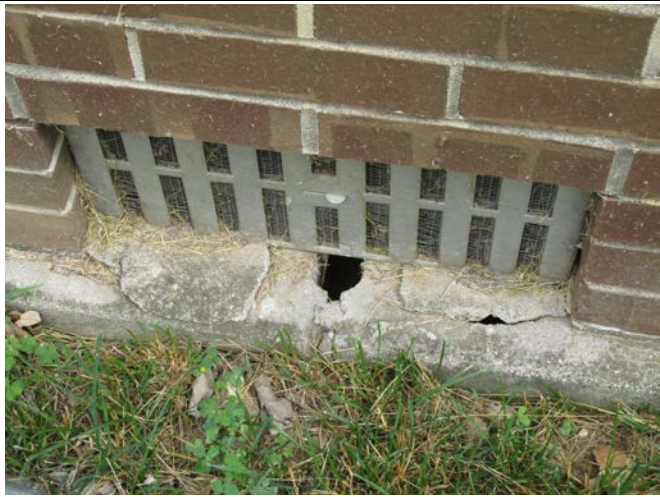
Photo 9 – Openings in Foundation at Crawl Space Vent
