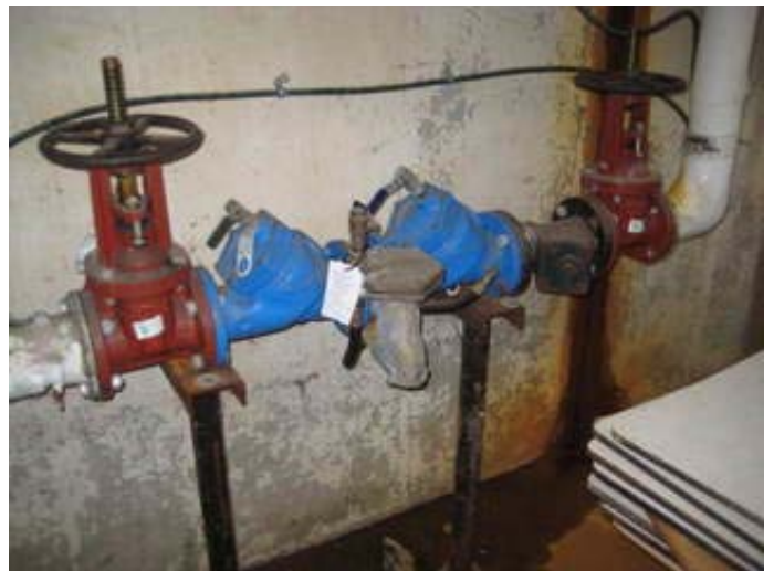
Incoming Domestic Water Service Meter
