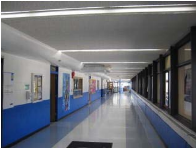
Typical Corridor Fluorescent Light Fixtures
