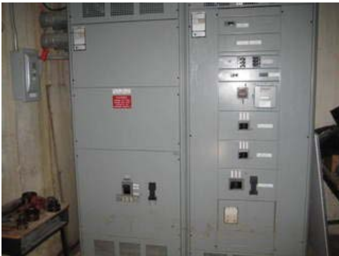
Main Electrical Distribution Panel
