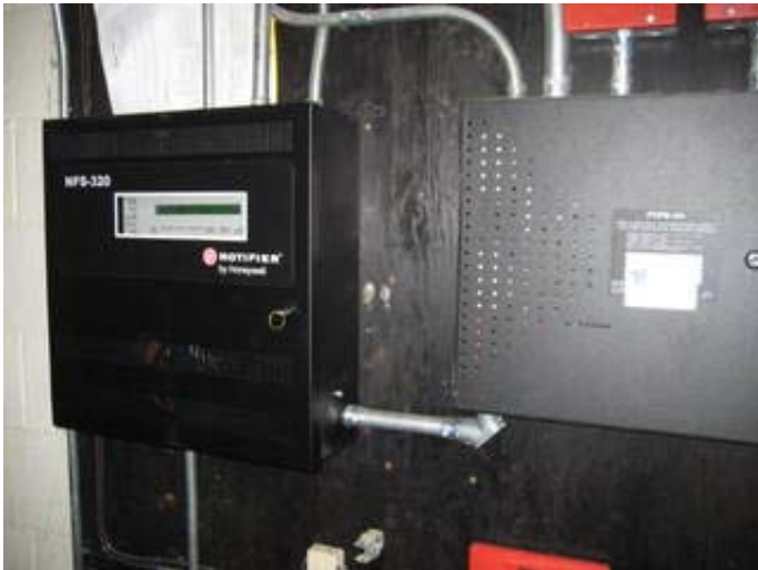
Fire Alarm System Control Panel
