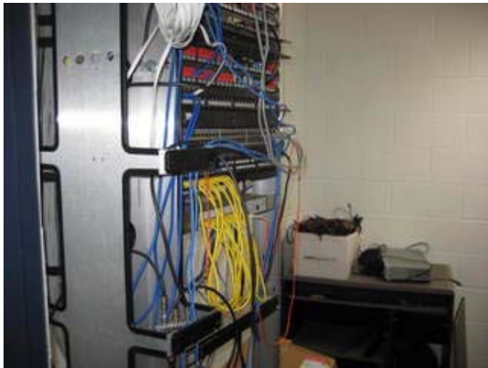
IT System Data Rack
