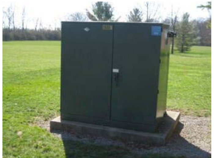
Pad Mounted Transformer
