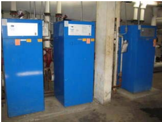
Natural Gas Fired Heated Water Boilers
