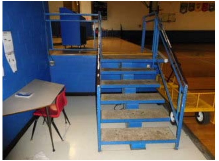
Non-ADA Compliant Stage Access
