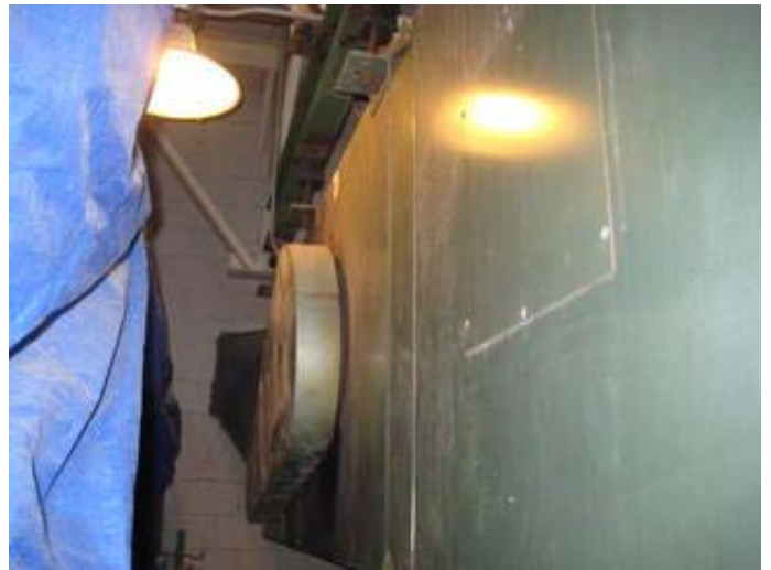
Service Area Incandescent Light Fixture
