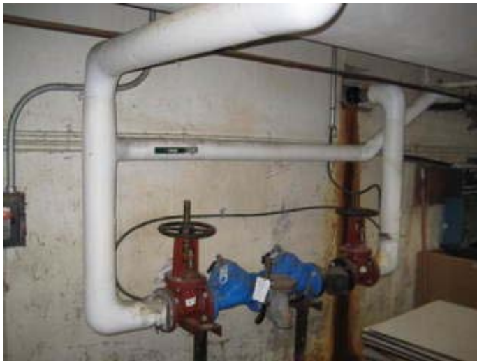
Incoming Domestic Water Service Line
