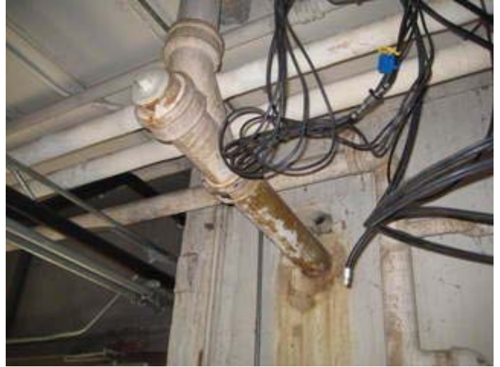
Sanitary Waste Piping
