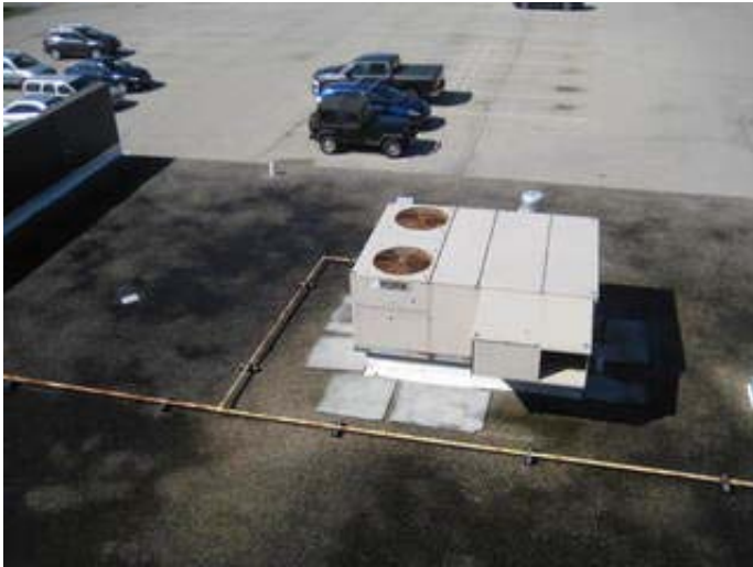
Roof Top Unit
