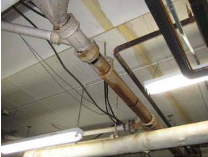
Sanitary Waste Piping
