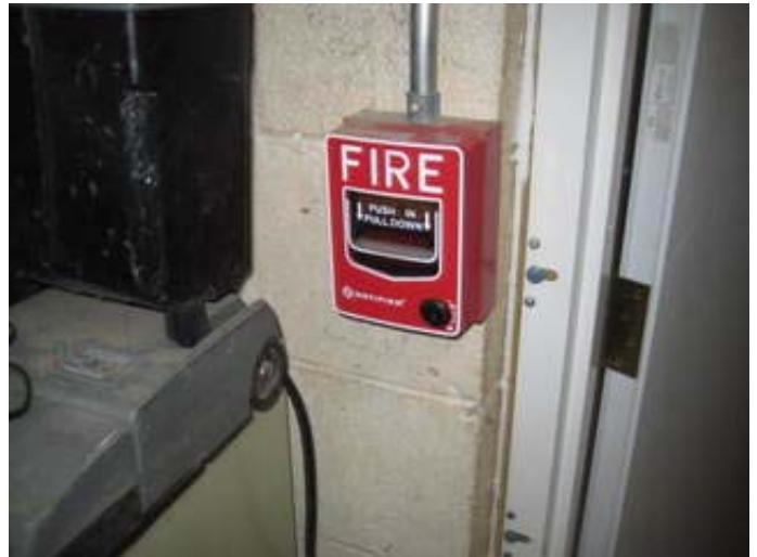
Fire Alarm System Manual Pull Station
