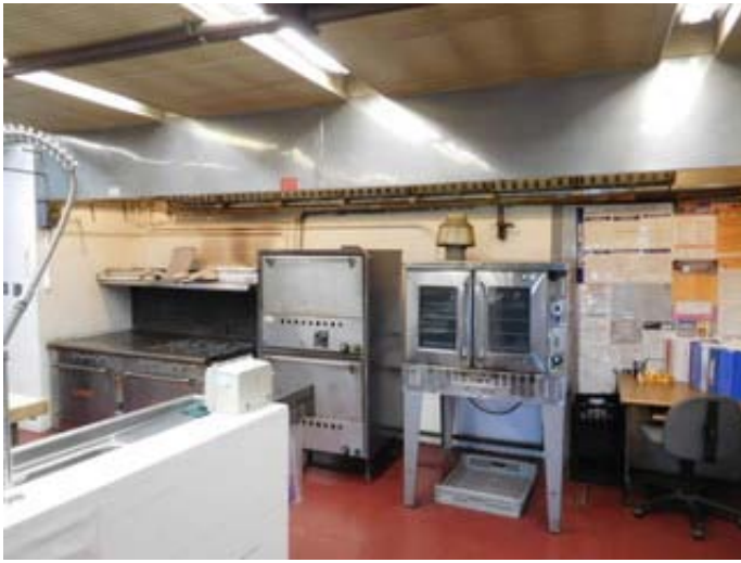
Kitchen Hood & Equipment
