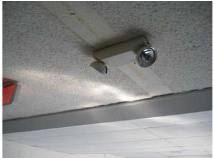
Emergency Egress Light Fixture
