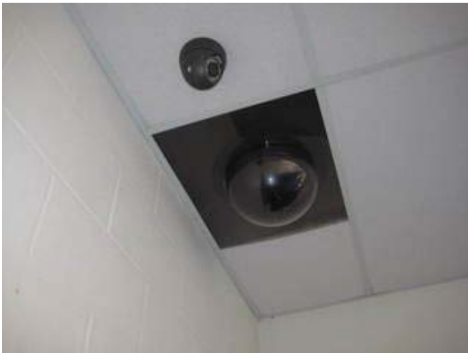
Security System CCTV Camera
