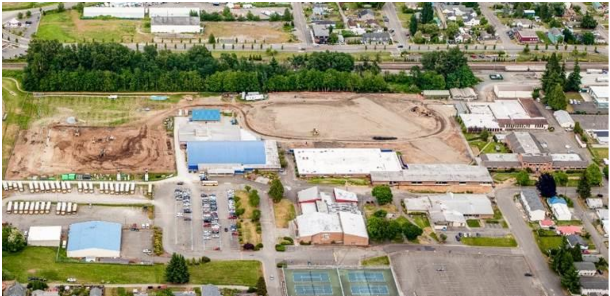
One year ago in June 2021, crews began preparations for the building pad. We have come a long way in one year!
