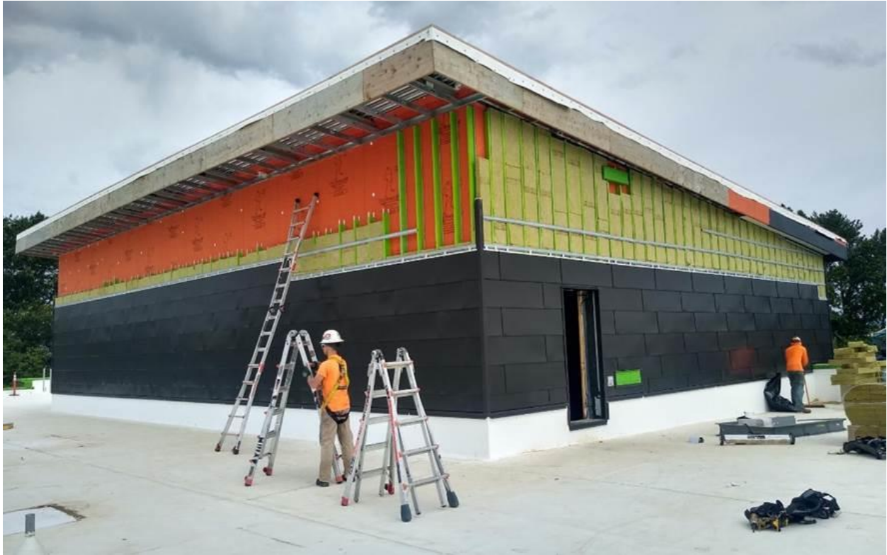
Final areas of siding being completed at the Academic Wing mechanical penthouses
