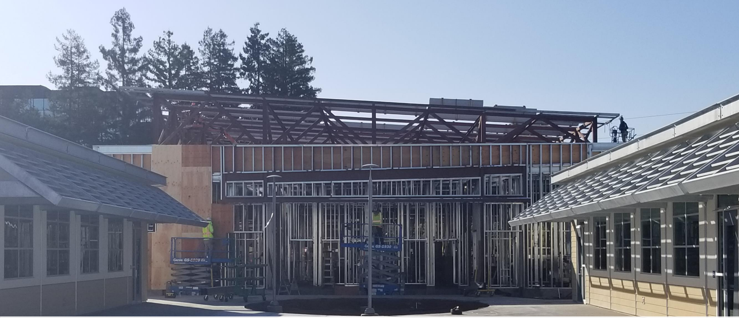
Borel--new classroom wings totaling 6 classrooms looking toward the entry to the locker rooms
