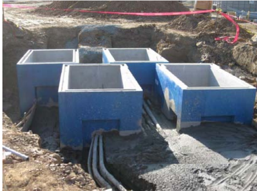
Courtyard Electrical Pull Boxes
