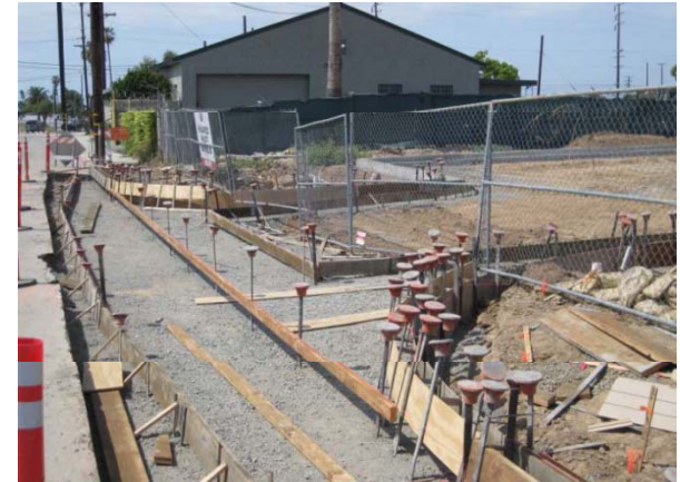
North Parking Lot Drive Approach
